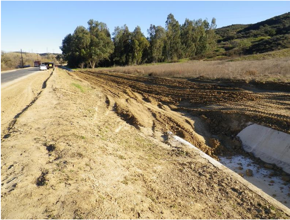
Figure 1: View showing the v-ditch after removal along the El Casco Substation access road. The photograph faces east.
