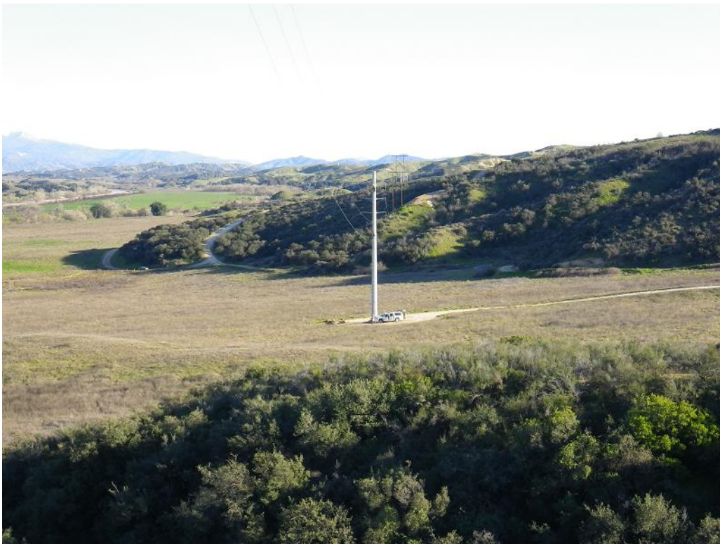
Figure 4: View of crews installing new poles just east of the El Casco Substation. The photograph faces east.
