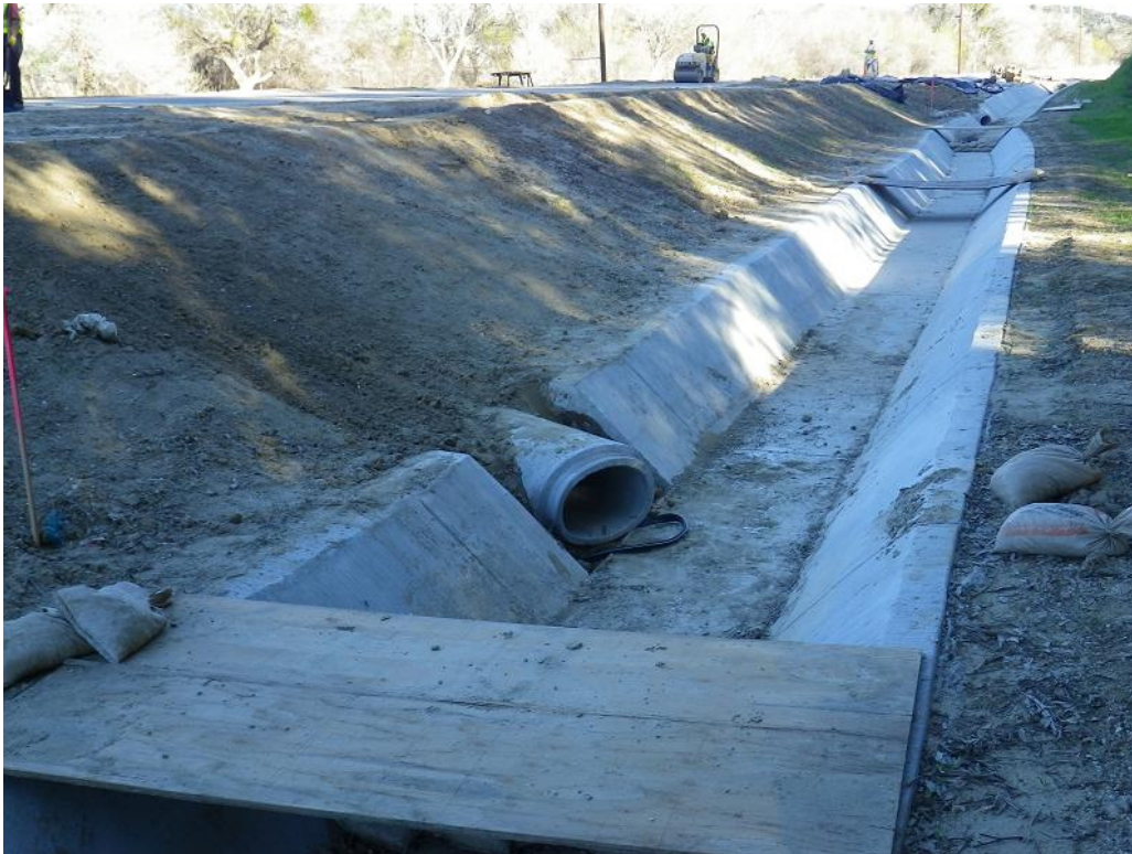
Figure 2: View of recently installed wildlife culverts under the main El Casco Substation access road. The photograph faces east.
