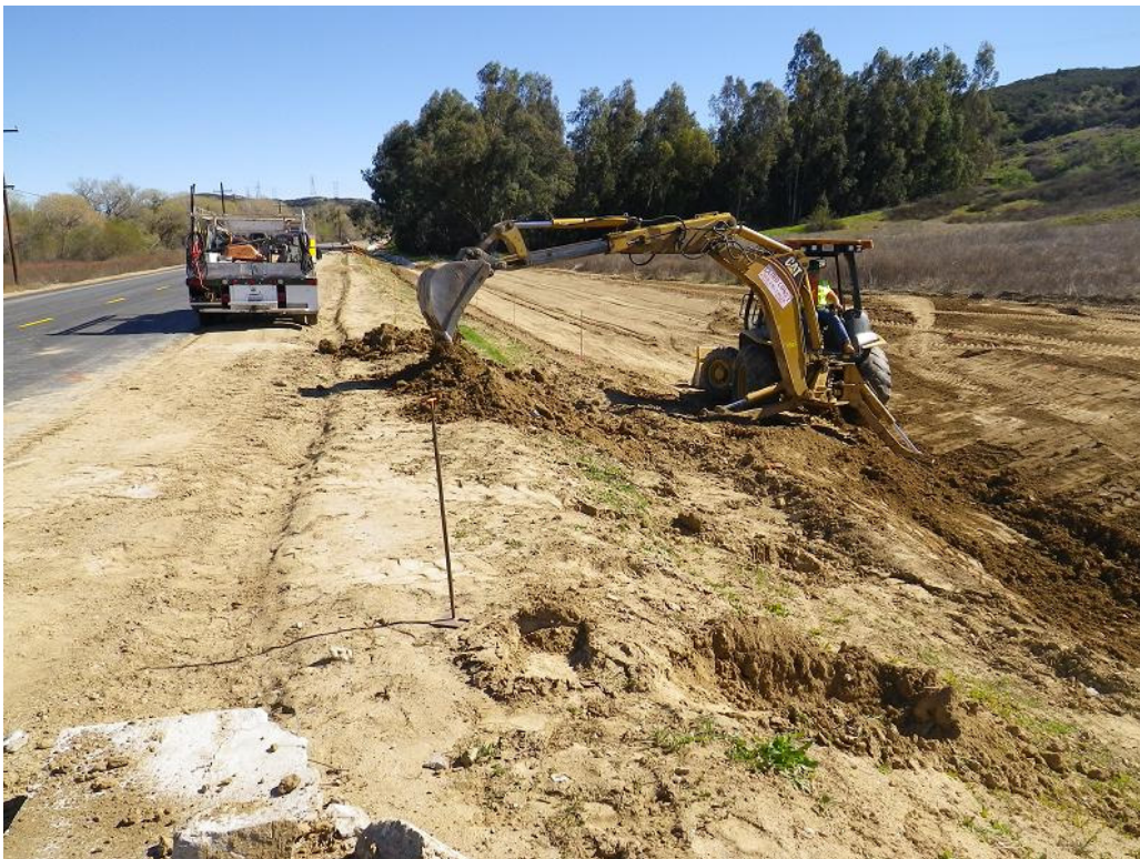
Figure 2: View of continued work on the v-ditches adjacent to the main El Casco Substation access road. The photograph faces east.
