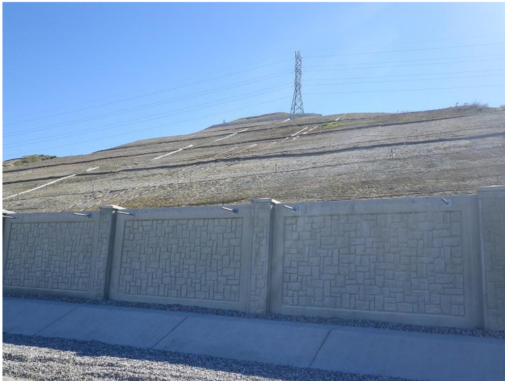
Figure 3: View of recently installed irrigation lines on the engineered slope just outside of the substation wall. The photograph faces south.
