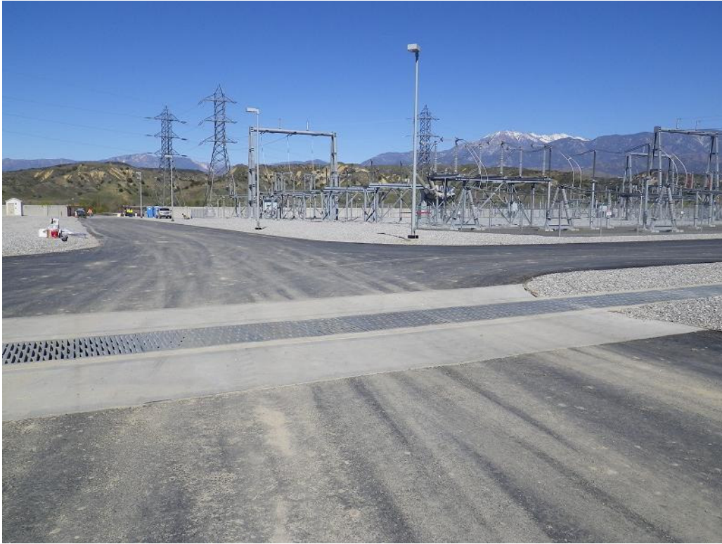
Figure 1: View showing the completed paved roads within the El Casco Substation. The photograph faces north.
