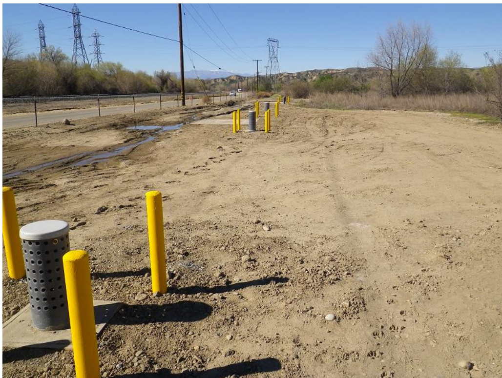
Figure 4: View of the HDD temporary work areas along San Timoteo Canyon Road. The photograph faces west.
