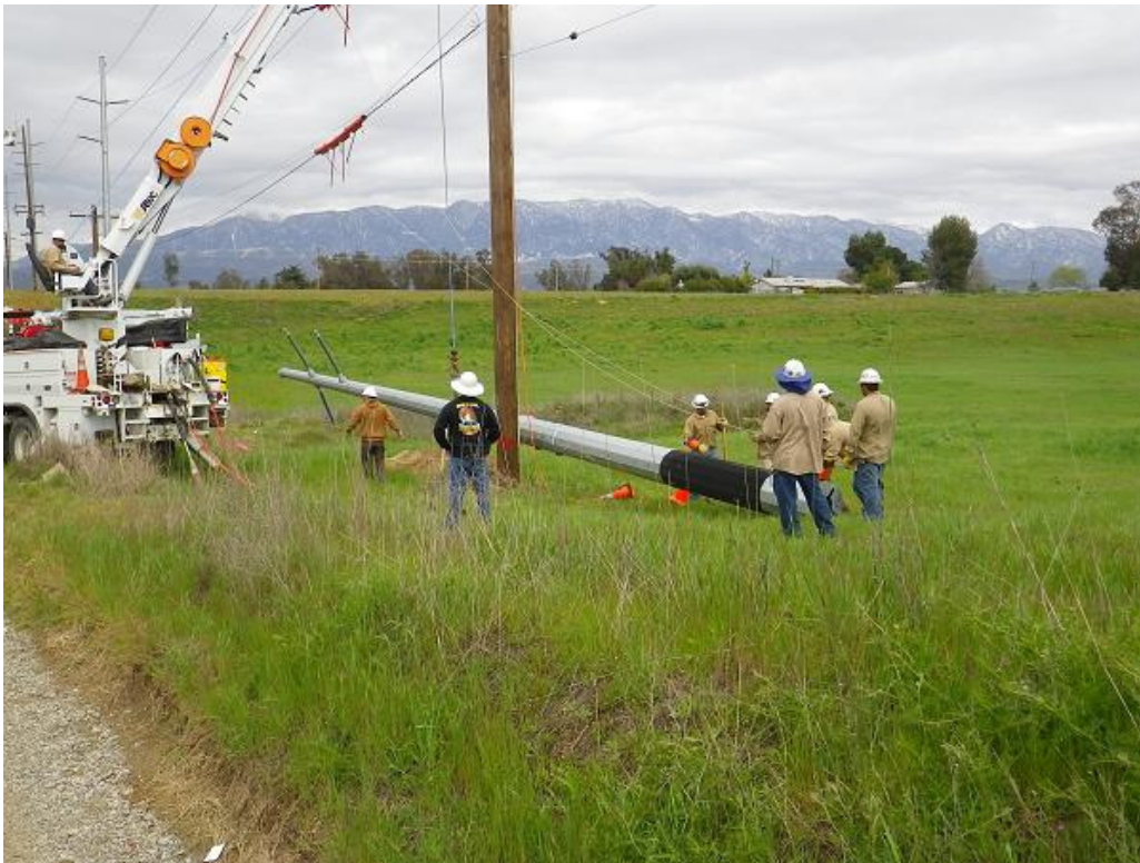
Figure 2: Crews installing poles along Veile Avenue, just south of Maraschino Substation, Segment 6 This photograph faces northeast.
