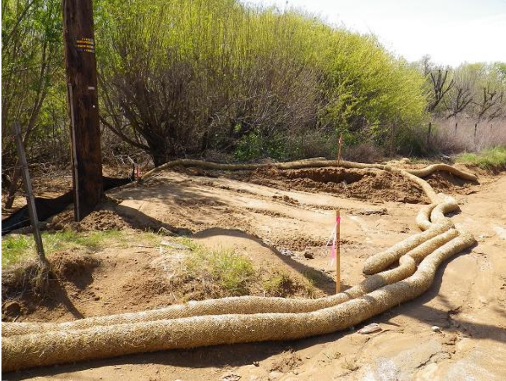
Figure 1: View of filled in foundation excavation at Pole 207 on Segment 7. The photograph faces west.
