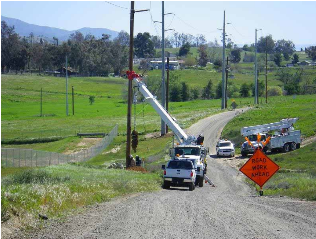
Figure 3: View of crews installing a pole on Segment 6. The photograph faces east.
