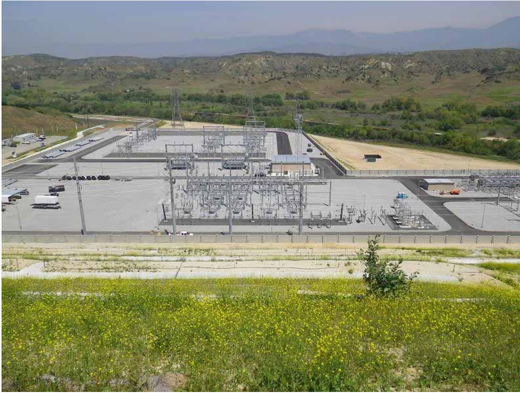
Figure 1: View of El Casco Substation. The photograph faces north.
