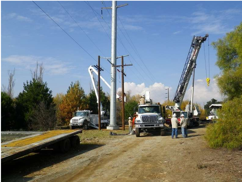
Figure 3: View of crews installing a pole along Segment 7, near the abandoned Christmas tree farm. The photograph faces northwest.
