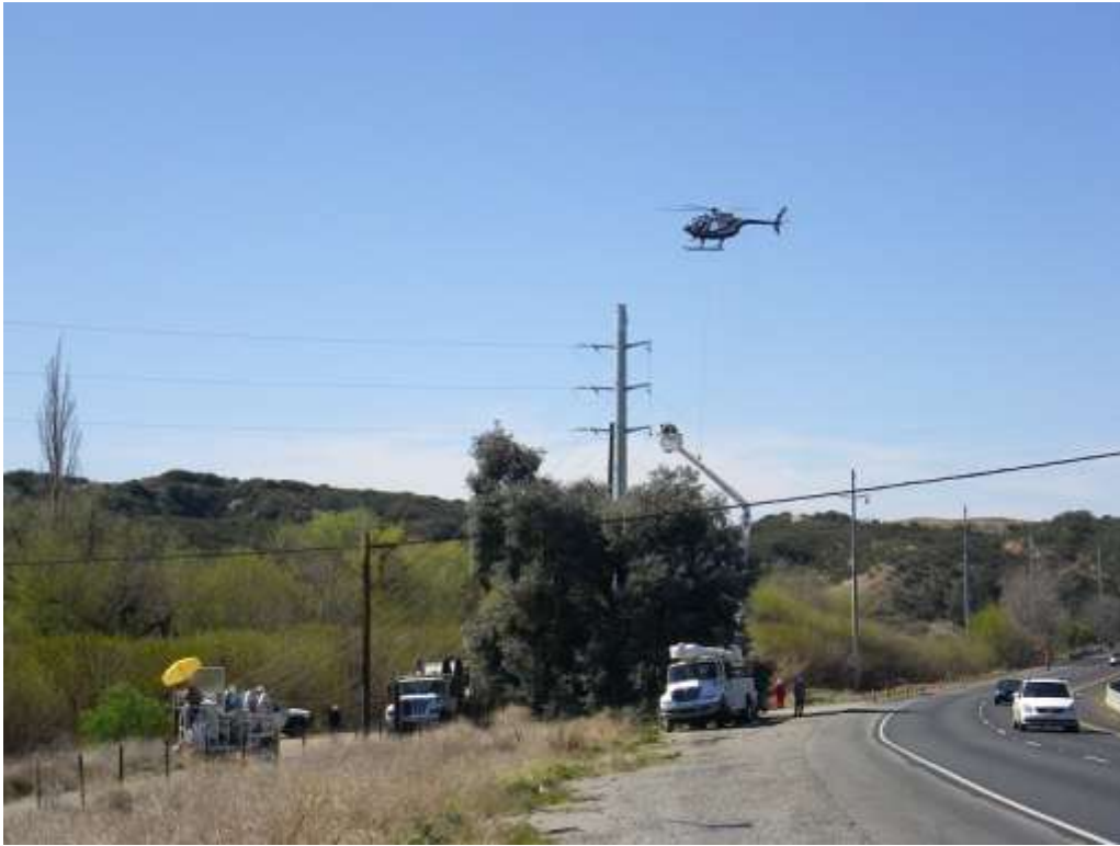
Figure 1: View of crews installing conductor along Segment 7 adjacent to Highway 60. The photograph faces west.
