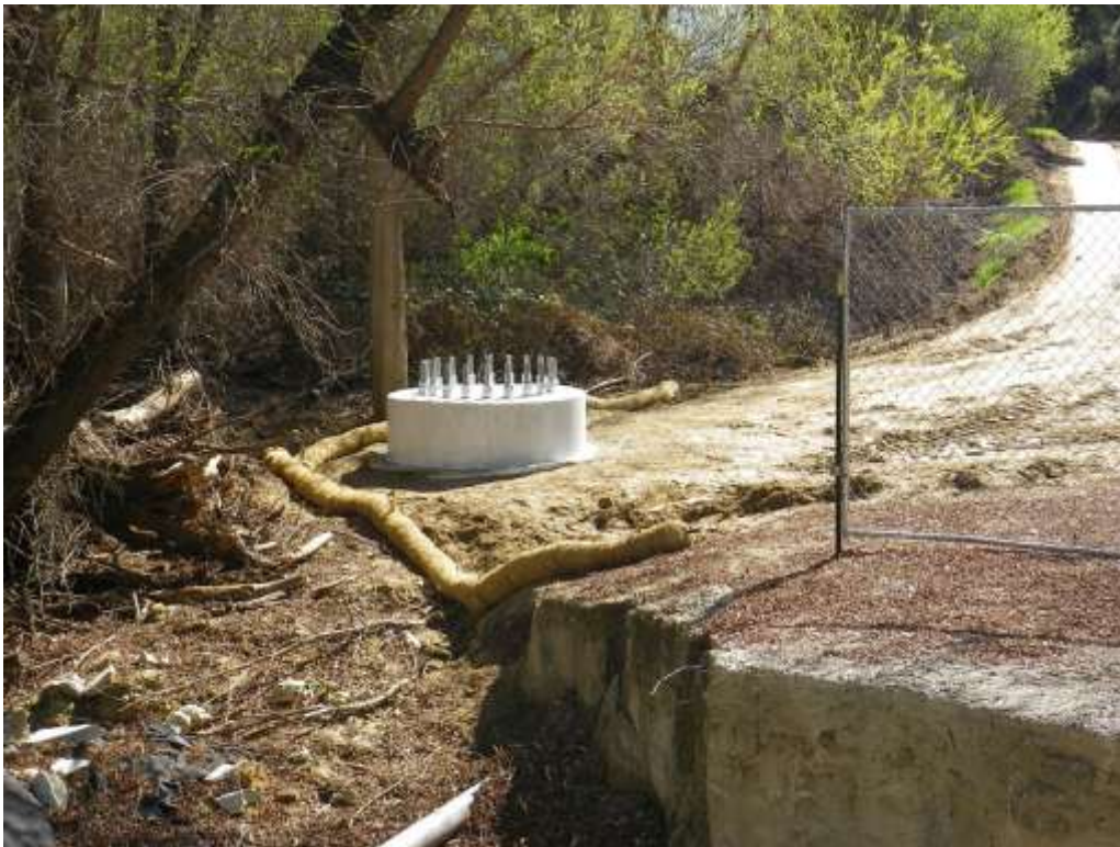
Figure 2: View of completed tubular steel pole foundation along Segment 5. The photograph faces southeast.
