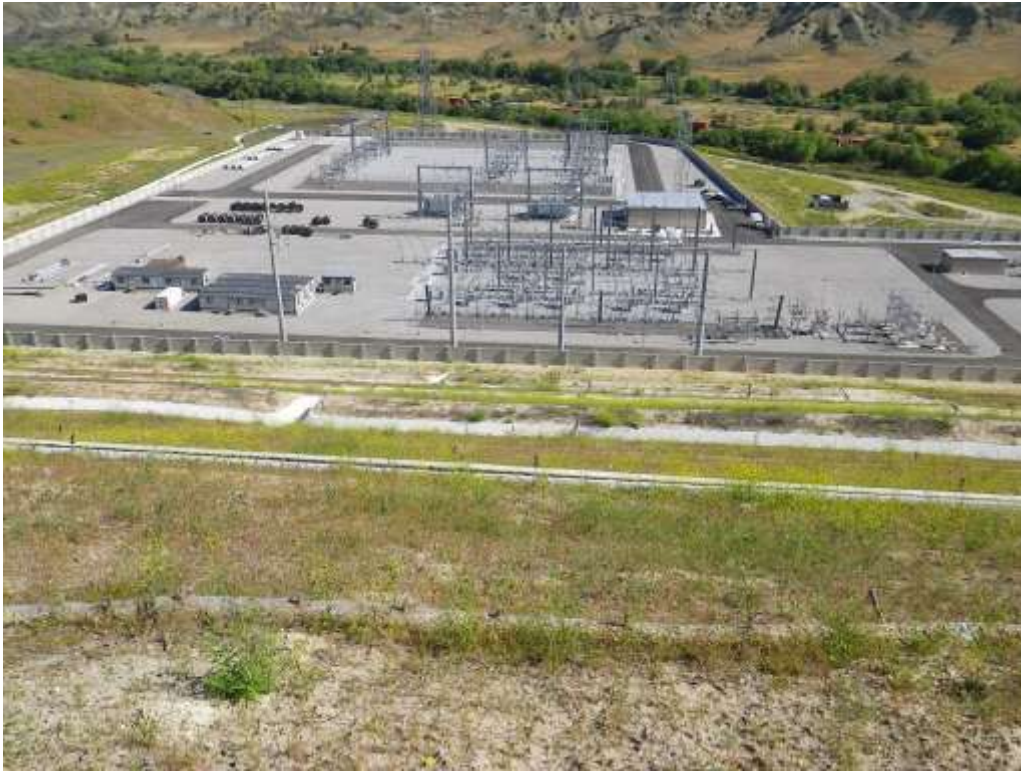
Figure 1: Overview of completed El Casco Substation. The photograph faces north.
