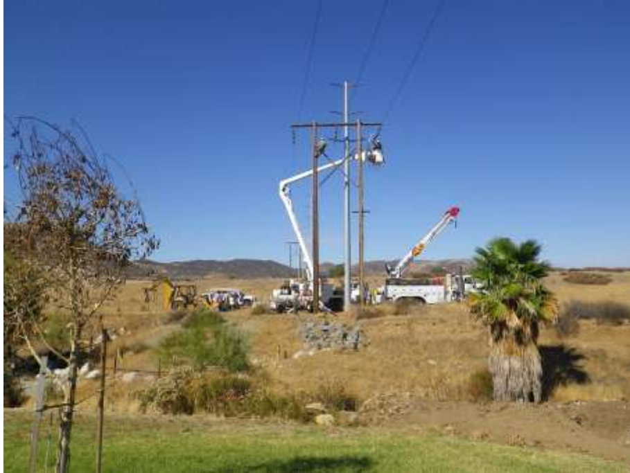
Figure 1: View of crews removing an old wooden pole from Segment 2 and rerouting the old conductor to the new steel pole. The photograph faces west.
