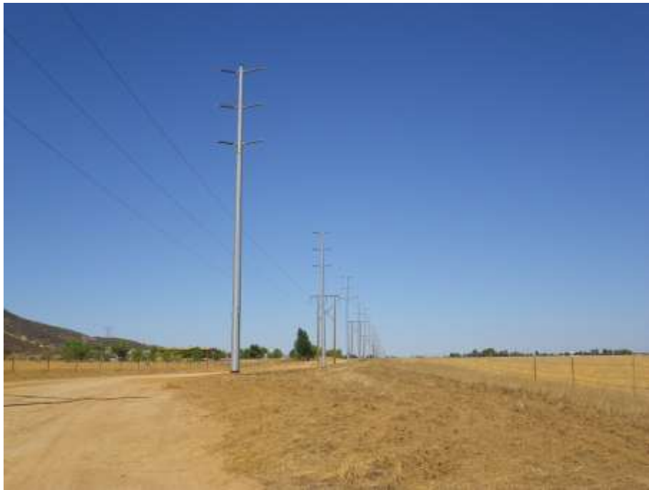
Figure 2: View of recently installed poles along a portion of Segment 2. Note that the old wooden poles have not yet been removed and the new conductor has not yet been installed. The photograph faces west.
