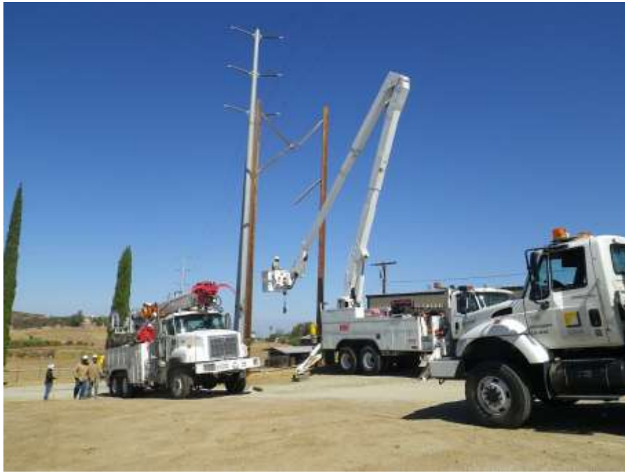
Figure 3: View of crews removing an old wooden pole along Segment 4, after the conductor had already been relocated to the new tubular steel pole. The photograph faces north.
