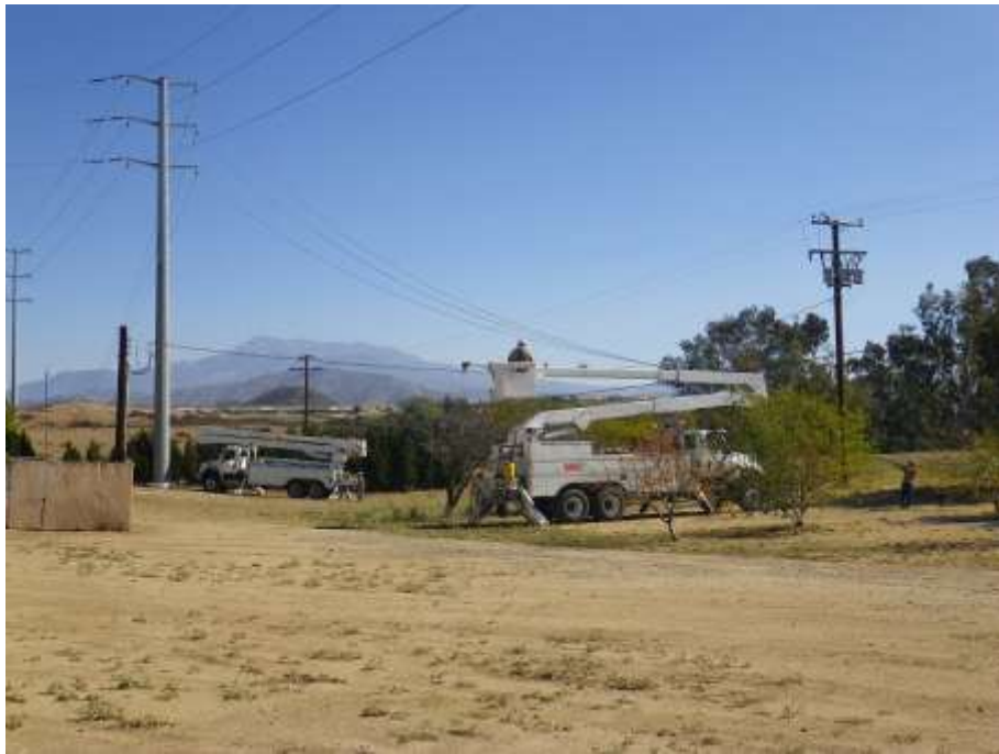
Figure 2: View of crews pulling new conductor on Segment 4. The photograph faces southeast.
