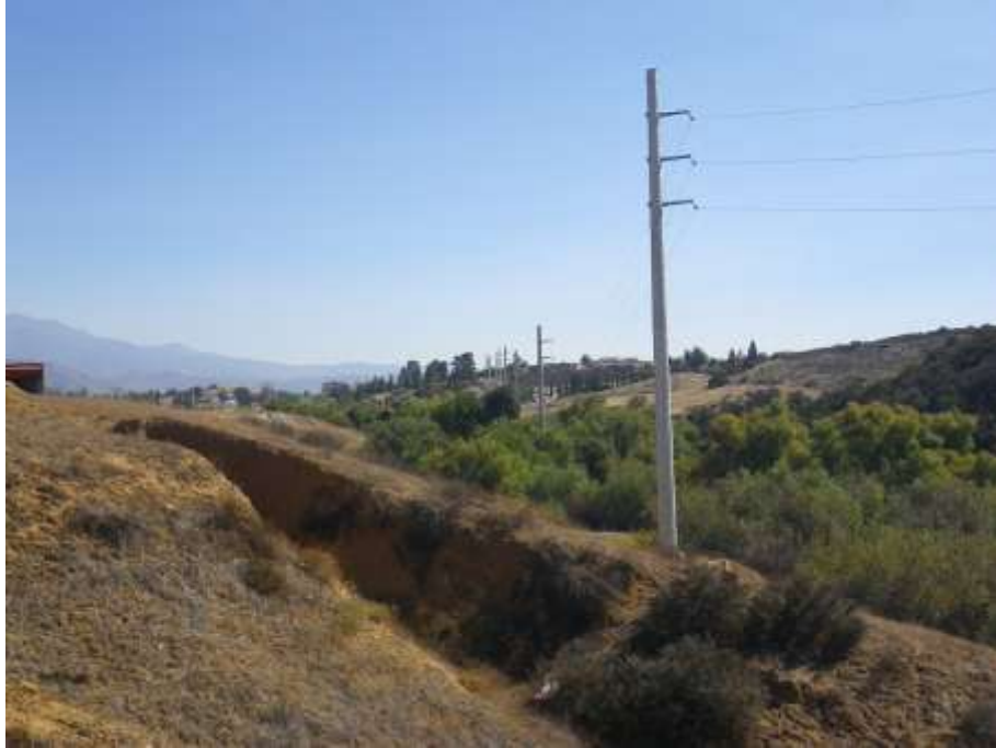
Figure 1: View of completed portion of Segment 5 crossing Smith Creek. The photograph faces southeast.
