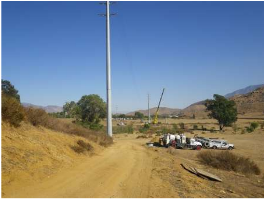
Figure 3: View of crews installing new steel poles on Segment 2 where the alignment crosses Montgomery Creek. The poles in the photo are the two temporary poles and the new pole can be seen in the background being lifted by a crane. The photograph faces east.
