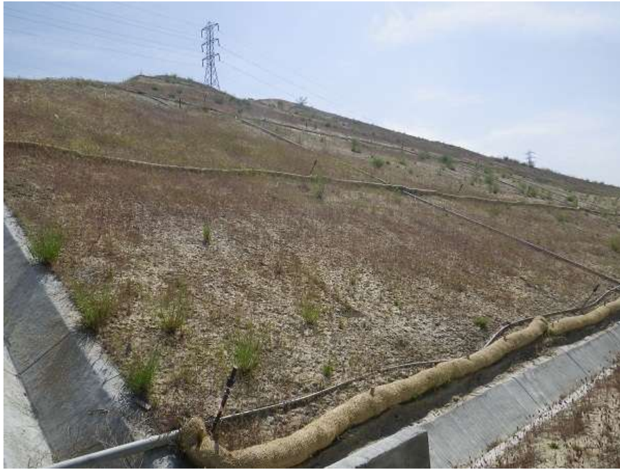
Figure 1: Southwest-facing view of the engineered slope behind the El Casco Substation. Photo taken: April 23, 2013.
