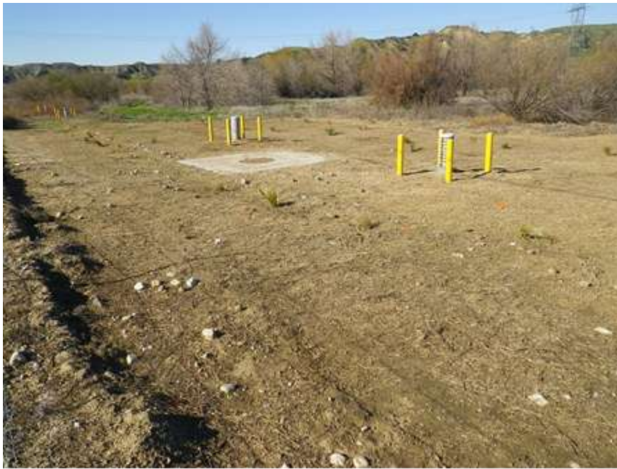
Figure 4: Northwest-facing view of the HDD restoration area. Several container plants were observed in the area and are marked by pin flags. Photo taken: February 11, 2013.
