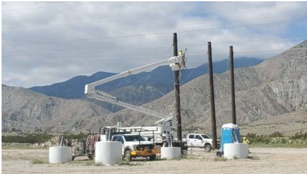
Photo 6 – Anchor installation at Construction Area 6X43, Segment 5 (March 24, 2020) (Photo courtesy of SCE).
