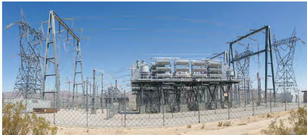
A capacitor bank (middle of photo) helps electricity to pass efficiently across long distances.
