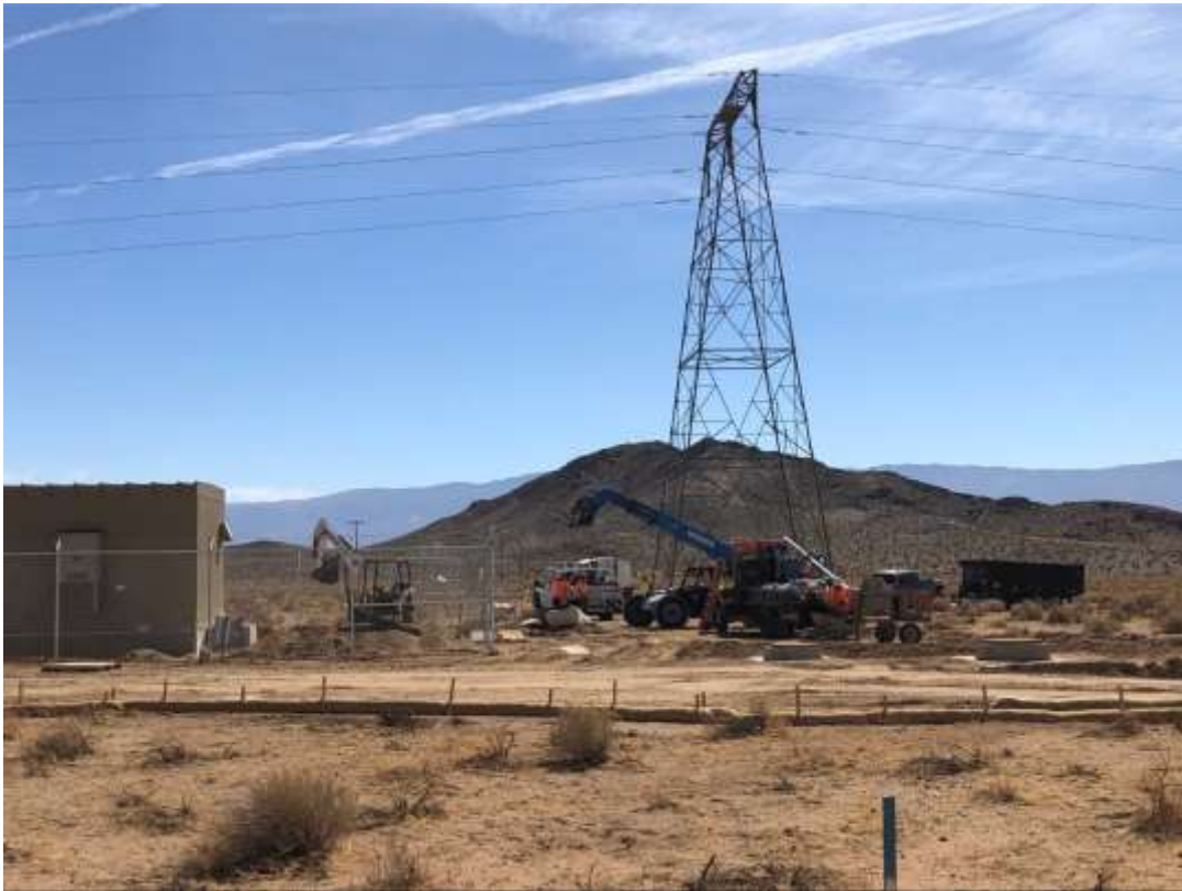
Photo 5: Development of Barstow Repeater (October 20, 2021).
