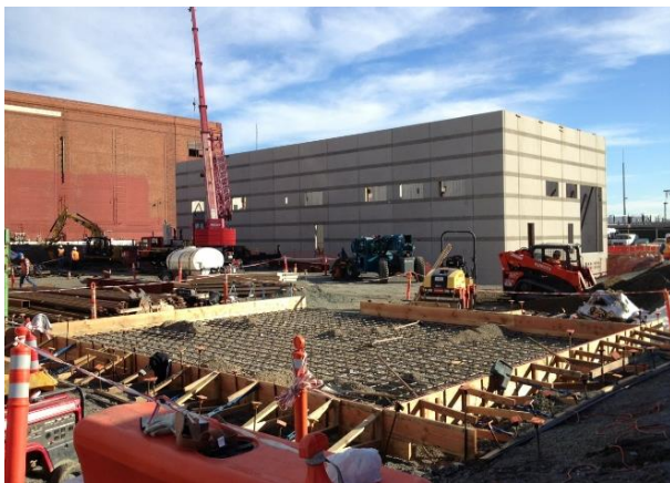
Figure 8. GIS building installation at Potrero Switchyard and reactor foundation in foreground, December 1, 2015
