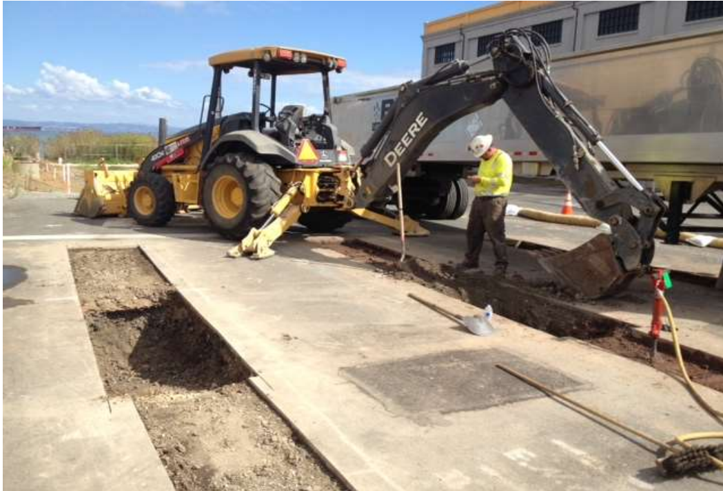
Figure 2 – HDD work activities on 23 rd Street excavating for casing installation. View east, September 18, 2014.
