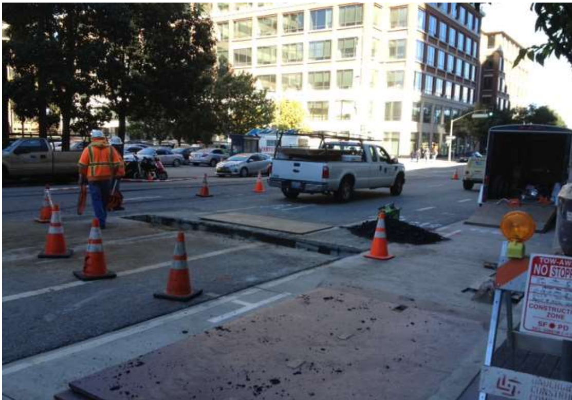
Figure 4 – Potholing for the underground duct bank on Folsom Street. View northwest, October 21, 2014.
