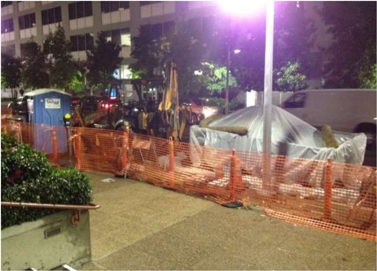
Figure 5 – 12 kV relocation equipment and materials staged on Spear Street. View southeast, November 20, 2014.
