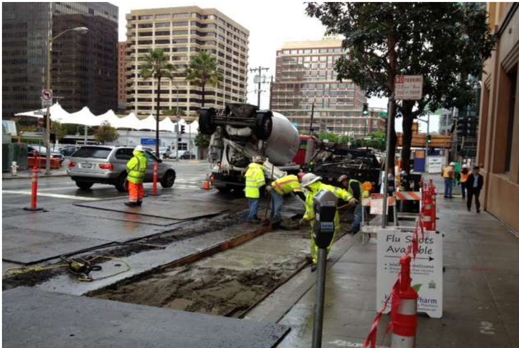
Figure 4 –Pouring cement slurry in duct bank trench on Folsom Street. View north, November 20, 2014.
