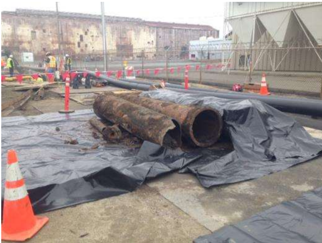
Figure 4 – Abandoned pipe removed at Duct Bank South. View north, December 9, 2014. (Photo courtesy of PG&E. )
