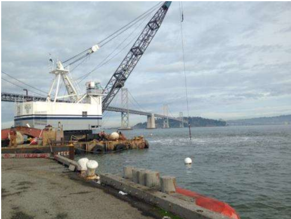
Figure 2 – Vortex conducting air lift at Bore 3 receiving pit at HDD North. View north, December 8, 2014. (Photo courtesy of PG&E.)
