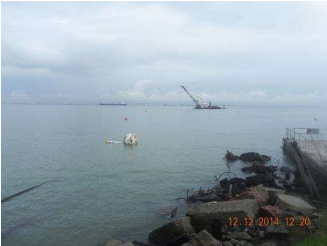
Figure 3 – Vortex staged to locate Bore 2 at receiving pit at HDD South. View southeast, December 12, 2014. (Photo courtesy of PG&E.)
