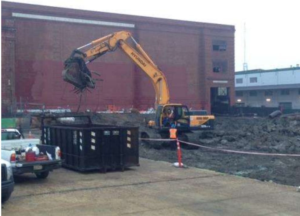
Figure 1 – Removal of rebar for recycling at Potrero Switchyard. View east-southeast, December 9, 2014. (Photo courtesy of PG&E.)
