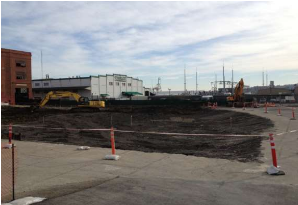
Figure 1 – Potrero Switchyard. View southeast, January 5, 2015.
