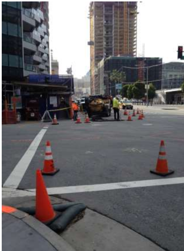
Figure 3 – Potholing for utilities at the corner of Folsom Street and Main Street. View southwest, January 5, 2015.
