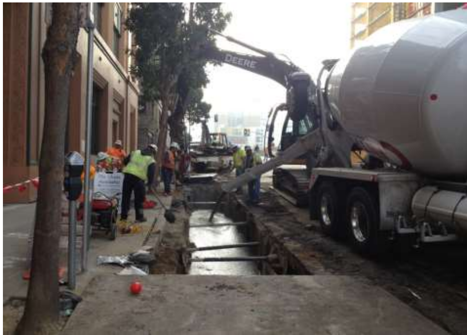
Figure 3 – Pouring cement slurry in duct bank trench on Folsom Street. View south-southwest, January 15, 2015.
