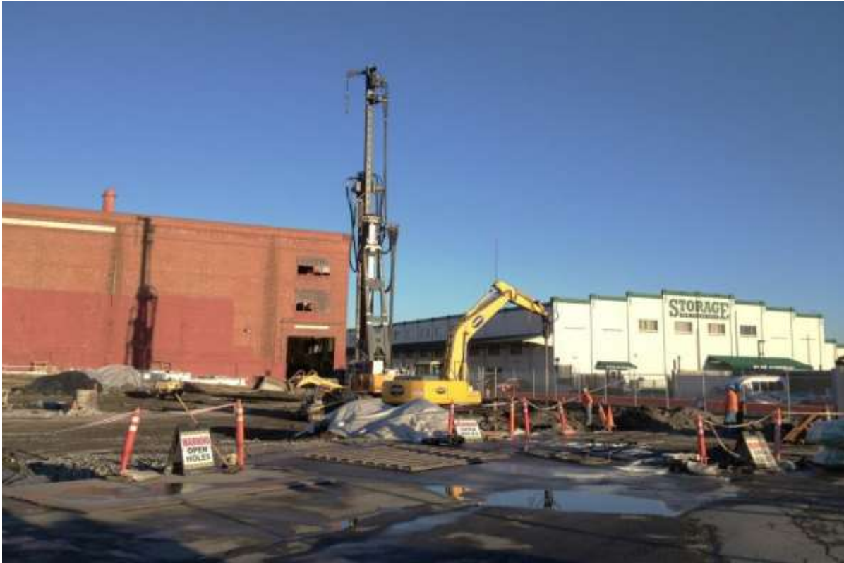
Figure 1 – Potrero Switchyard, view southeast, February 20, 2015.
