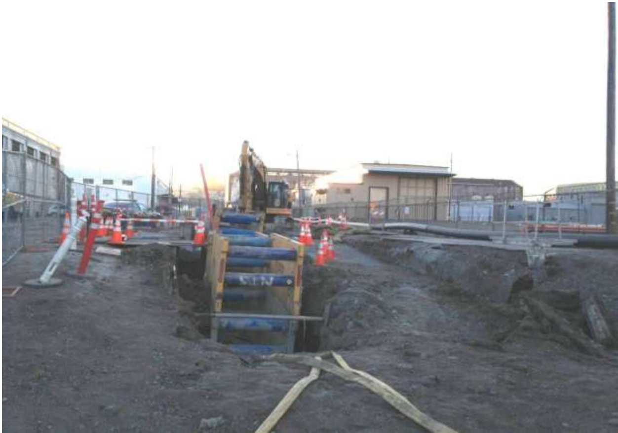
Figure 5 – Duct Bank South trench shored on 23 rd Street and surrounded by chain link fence. View west, February 20, 2015.
