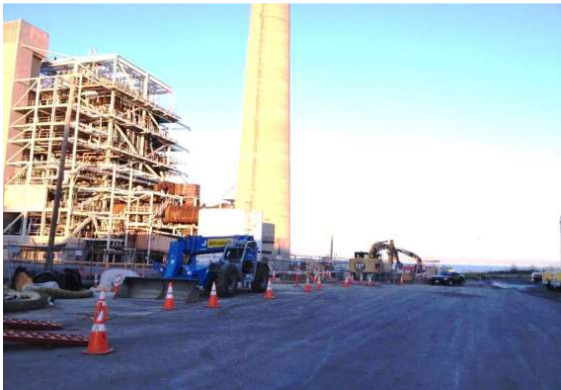
Figure 4 – Work area at Duct Bank South on 23 rd Street. View east, February 20, 2015.
