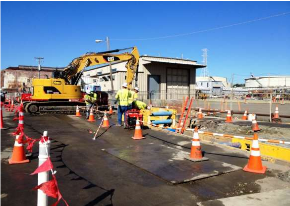
Figure 4 – Underground conduit tie-in work in duct bank at Bore 1 on 23 rd Street. View northwest, March 4, 2015.
