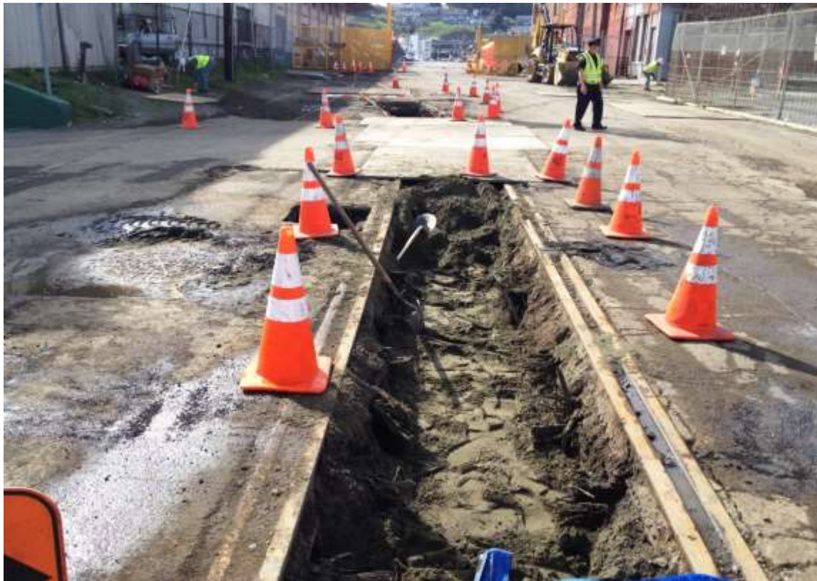
Figure 4 – Underground duct bank and water line relocation work on 23 rd Street. View west, March 12, 2015.
