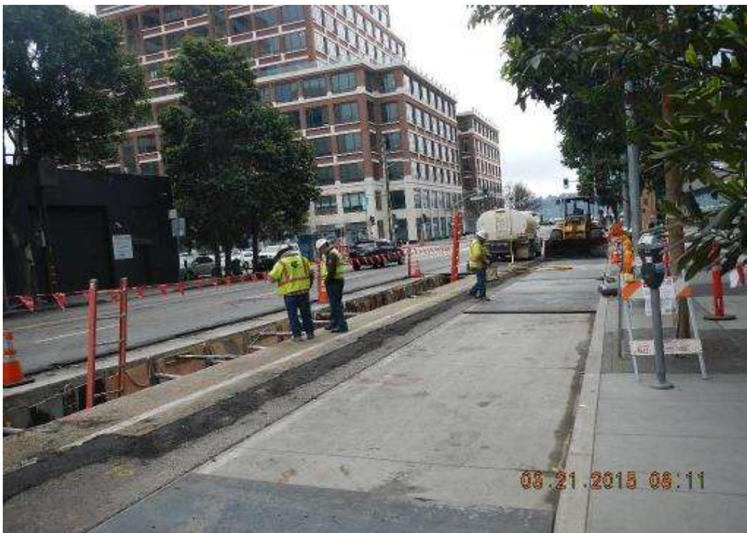
Figure 2 – Dewatering and installing rebar in duct bank on Folsom Street. View north, March 21, 2015. Photo courtesy of PG&E.
