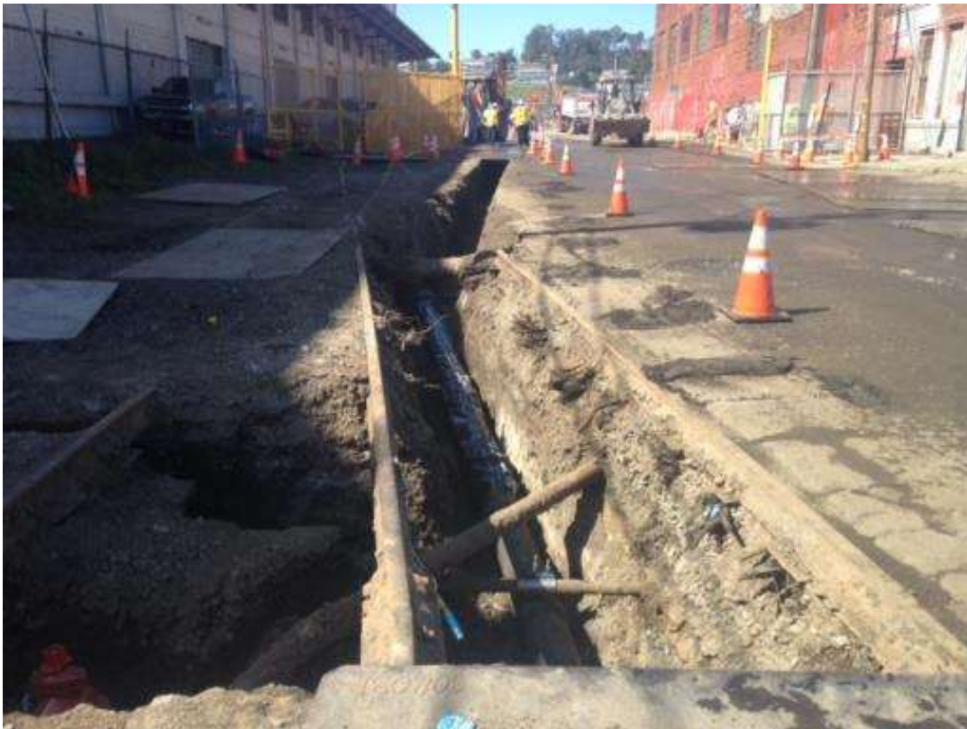
Figure 4 – Underground duct bank and water line relocation work on 23 rd Street. View west, March 18, 2015. Photo courtesy of PG&E.
