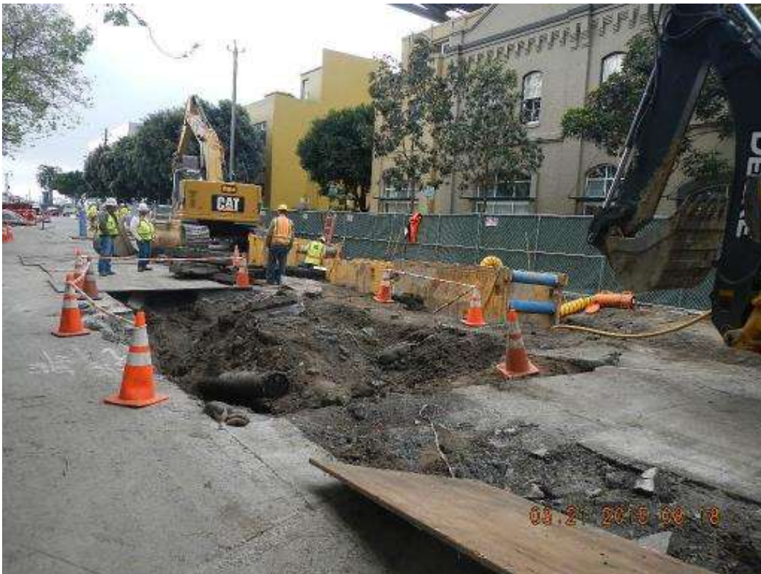
Figure 3 – Excavating for duct bank at the HDPE transition on Spear Street. View east, March 21, 2015. Photo courtesy of PG&E.
