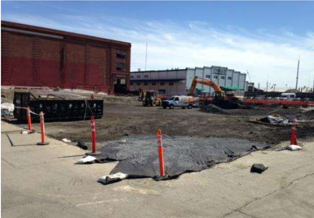
Figure 1 – New access ramp into work area being built at Potrero Switchyard, view southeast, March 17, 2015. Photo courtesy of PG&E.
