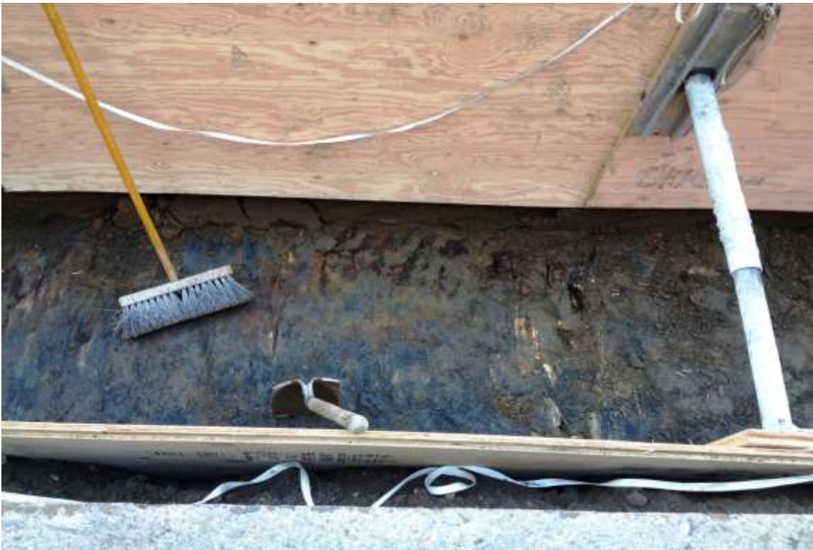
Figure 3 – Remnants of old pier structure on Folsom Street. View west, March 25, 2015.
