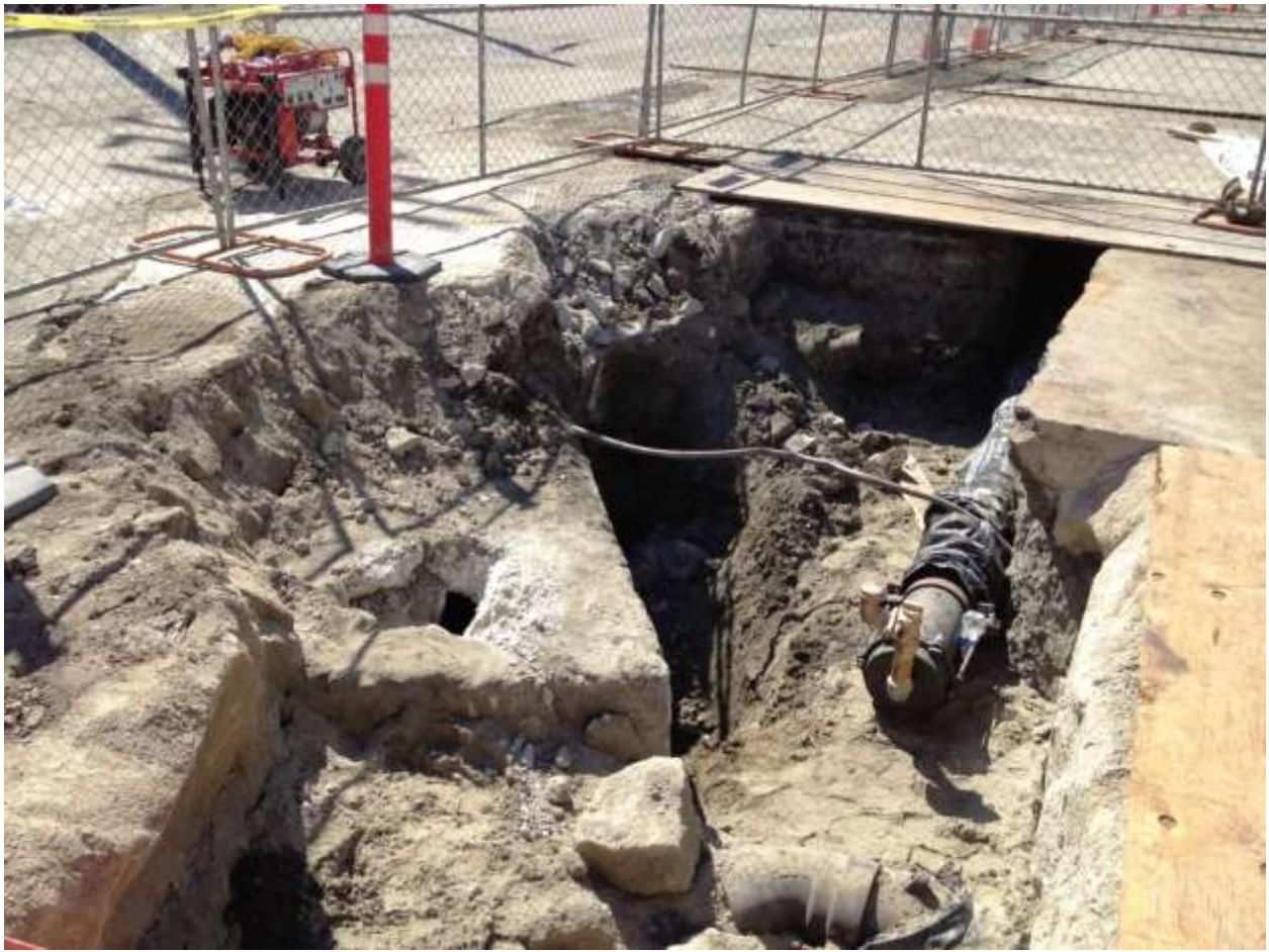
Figure 5 – Second room of underground water circulation feature exposed on 23 rd Street. View southwest, March 25, 2015.
