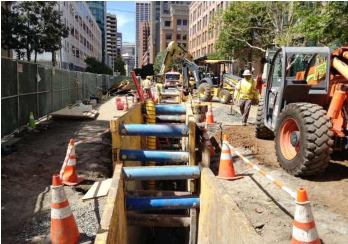
Figure 3 – HDPE conduit connection at HDD Bore 2 transition on Spear Street. View west, April 9, 2015.
