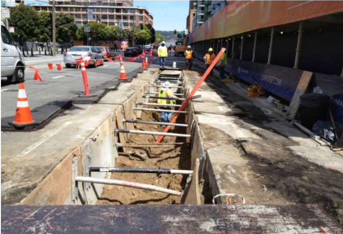
Figure 1 – Potholing from within the trench on Folsom Street just north of Beale Street, view north, April 9, 2015.
