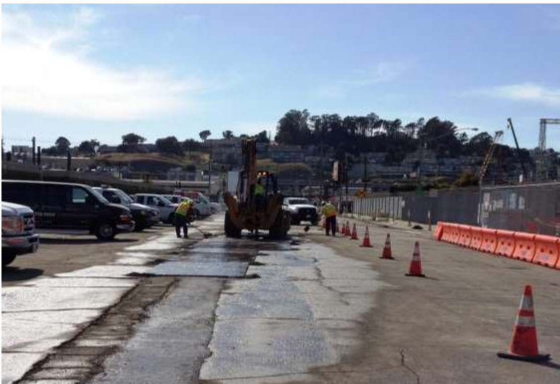
Figure 4 – Plating waterline trench at the end of the day and watering road on 23 rd Street. View west, April 9, 2015.
