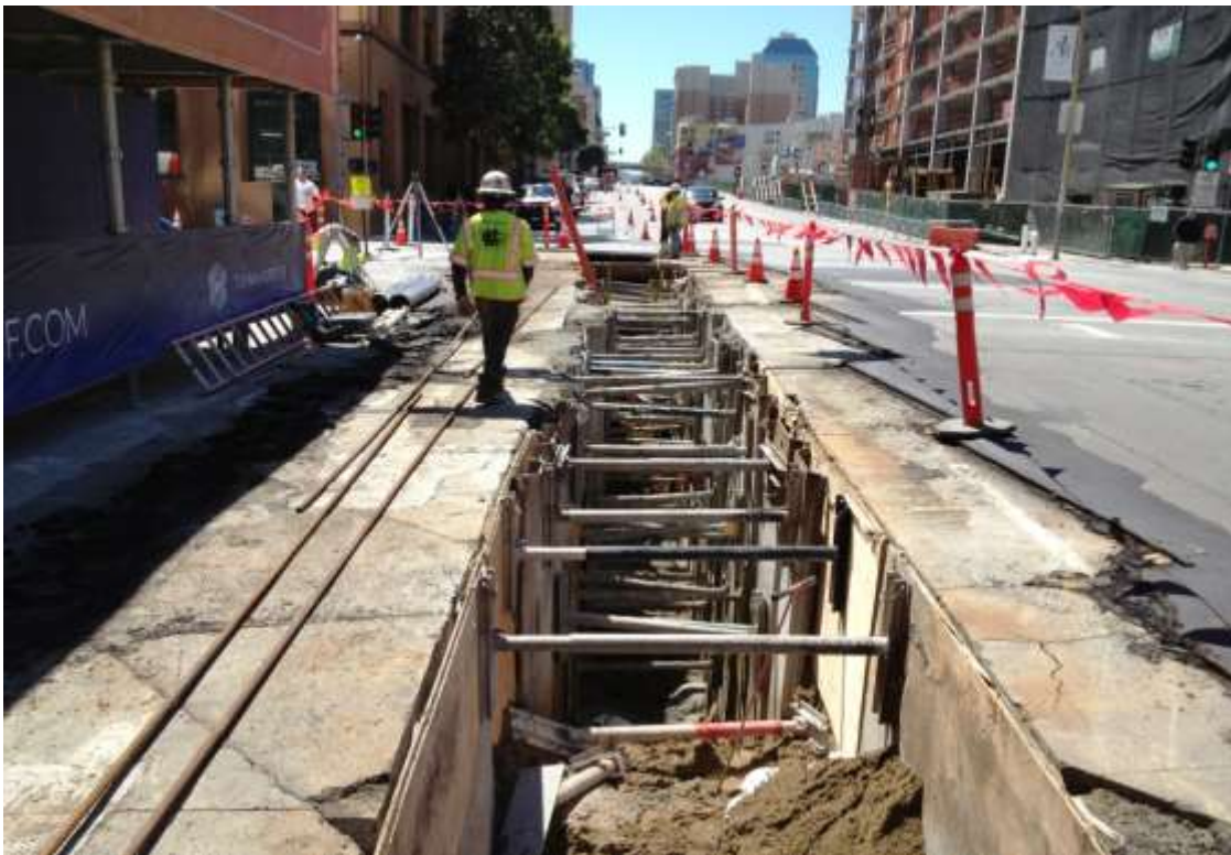
Figure 2 – Duct bank work on Folsom Street between Beale Street and Main Street. View south, April 14, 2015.
