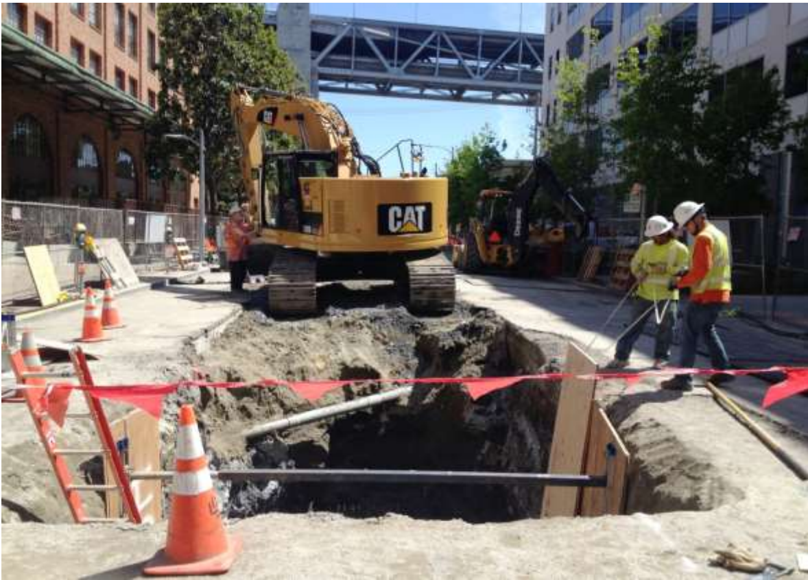
Figure 3 – Excavating on east side of vault for tie-in on Spear Street. View east, April 14, 2015.
