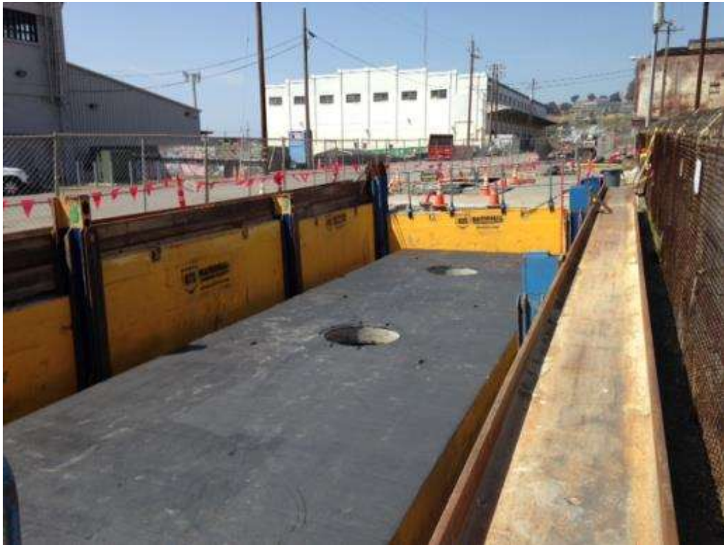
Figure 3 – Vault after sides and top were installed on 23 rd Street for the underground duct bank. View west, April 23, 2015. Photo courtesy of PG&E.
