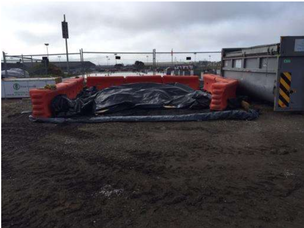
Figure 4 – Cutback stockpile properly covered and contained at Amador Yard. View south, April 25, 2015. Photo courtesy of PG&E.
