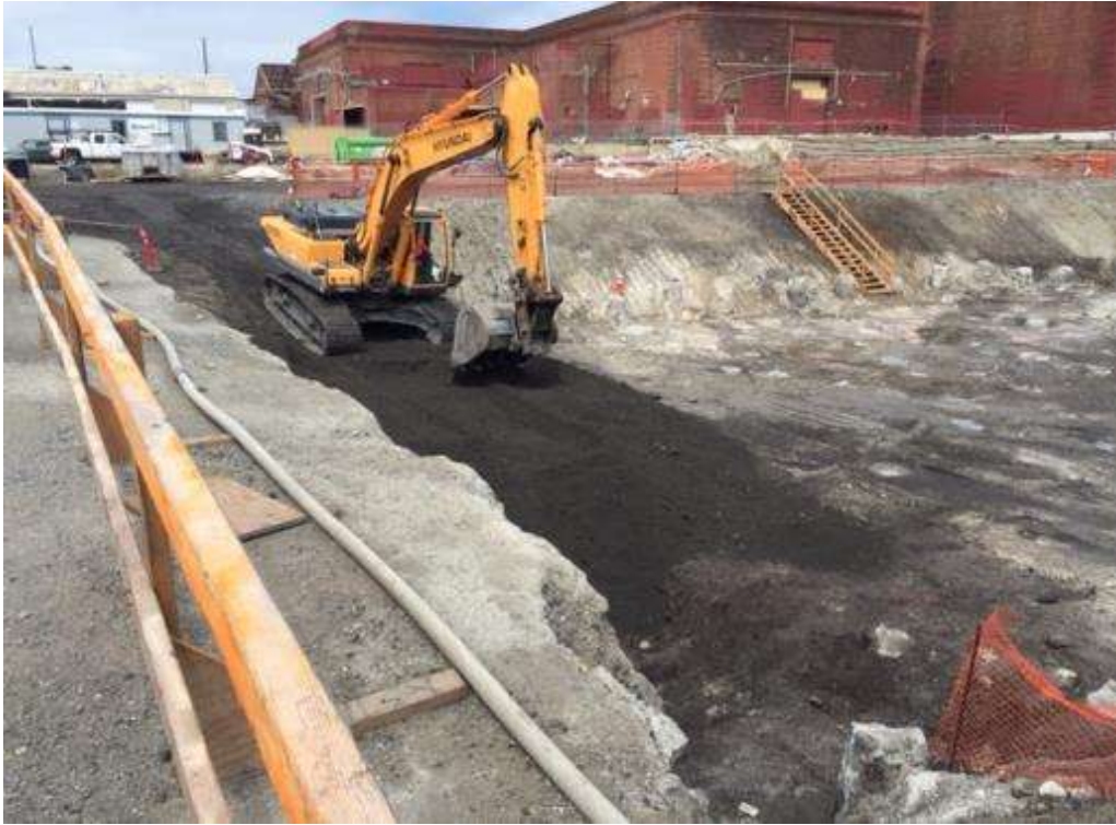
Figure 1 – Proven backfilling excavation at Potrero Switchyard. View northeast, April 20, 2015. Photo courtesy of PG&E.
