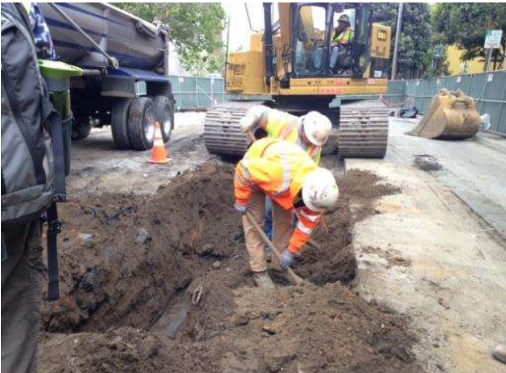
Figure 2 – Hand excavating at N1 for HDPE transition on Spear Street where possible pier structure has been encountered. View east, April 21, 2015. Photo courtesy of PG&E.
