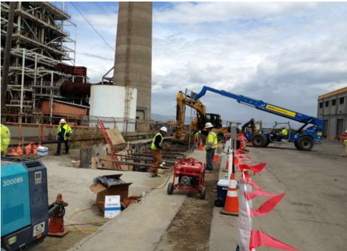
Figure 4 – Installing conduit in duct bank trench on 23 rd Street east of vault. View east, May 7, 2015.
