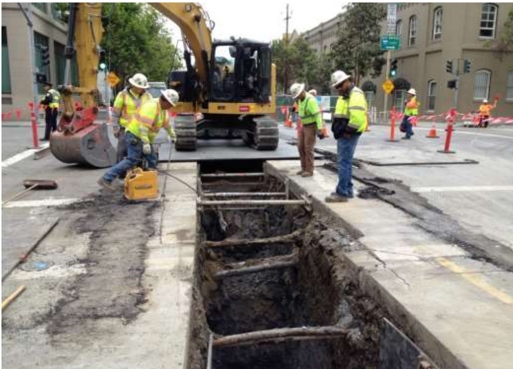
Figure 2 – Excavating duct bank trench on Spear Street east of vault. View east, May 7, 2015.
