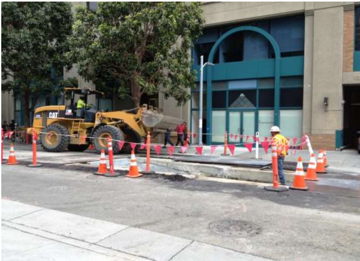
Figure 3 – Backfilling around pull box on Spear St. west of vault. View north, May 7, 2015.
