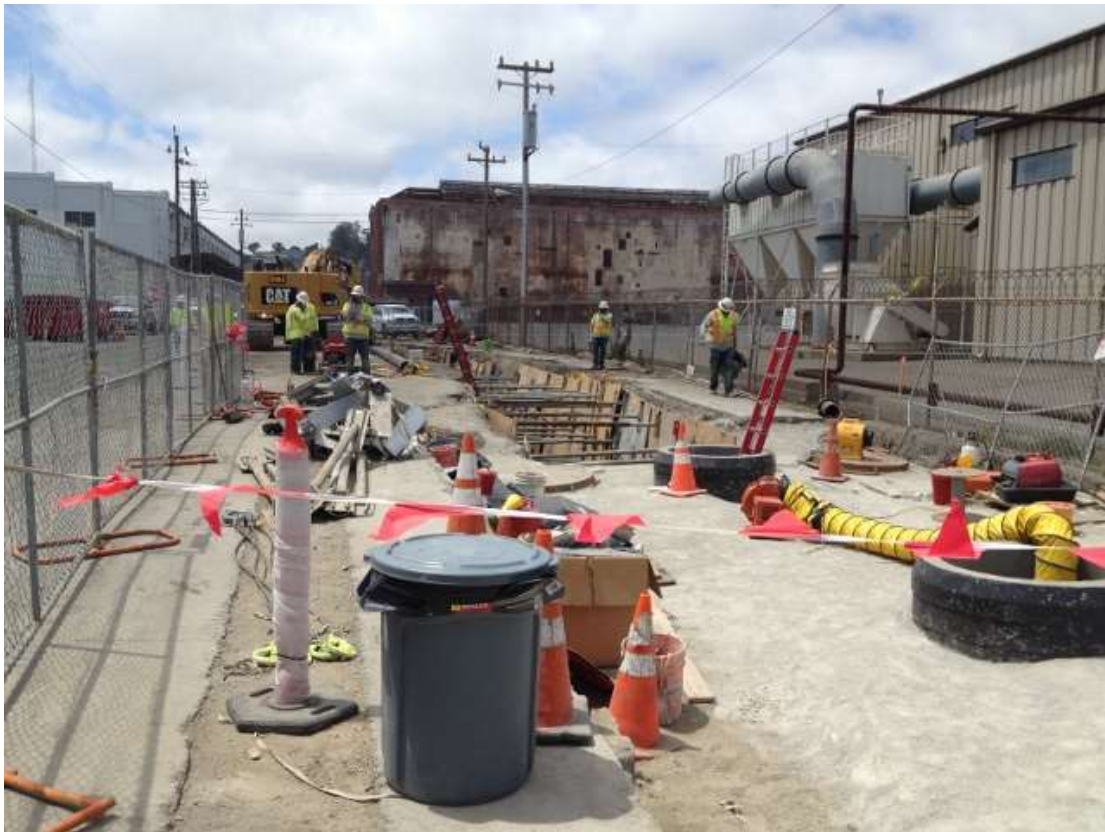
Figure 3 – Installed HDPE conduit on west side of vault on 23 rd Street. View west, May 15, 2015.
