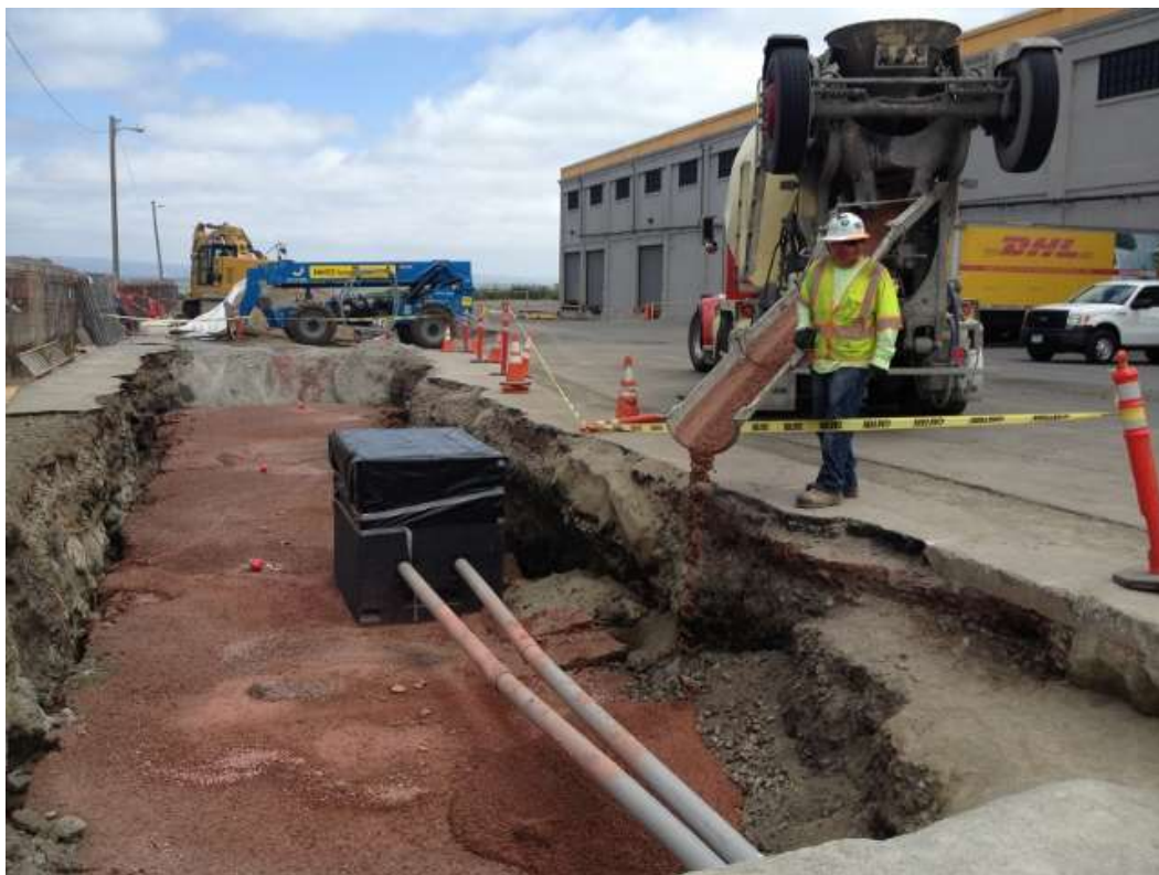
Figure 4 – Backfilling with FTB in duct bank trench on east side of vault on 23 rd St. View east, May 15, 2015.
