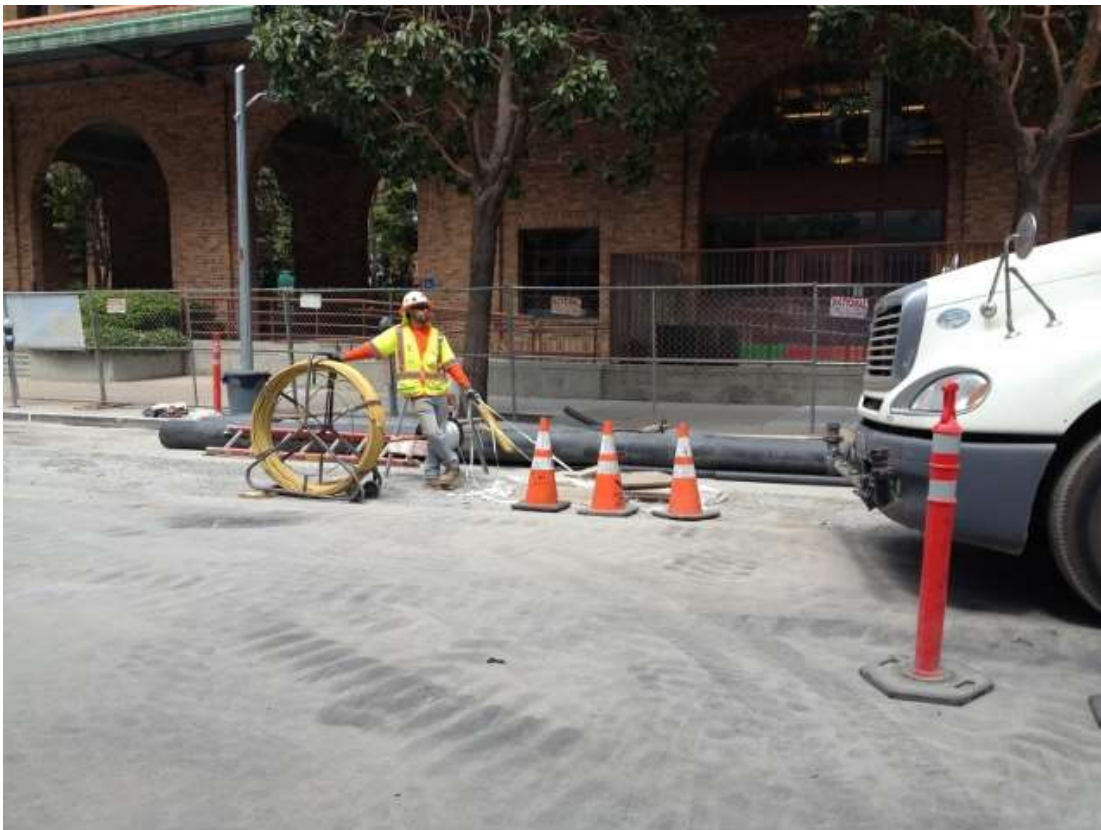
Figure 2 – Installing mule tape in fiber optic conduit on Spear Street. View north, May 15, 2015.
