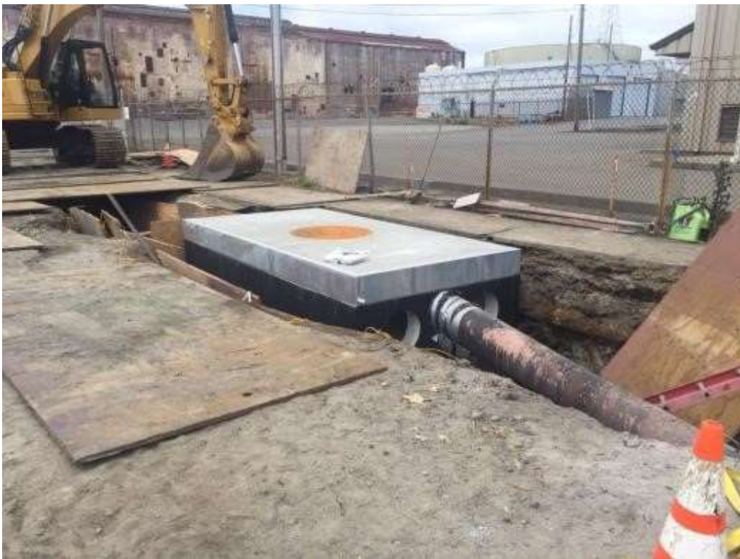
Figure 4 – Installed pull box cover at duct bank south on 23 rd St. View northwest, May 21, 2015. Photo courtesy of PG&E.
