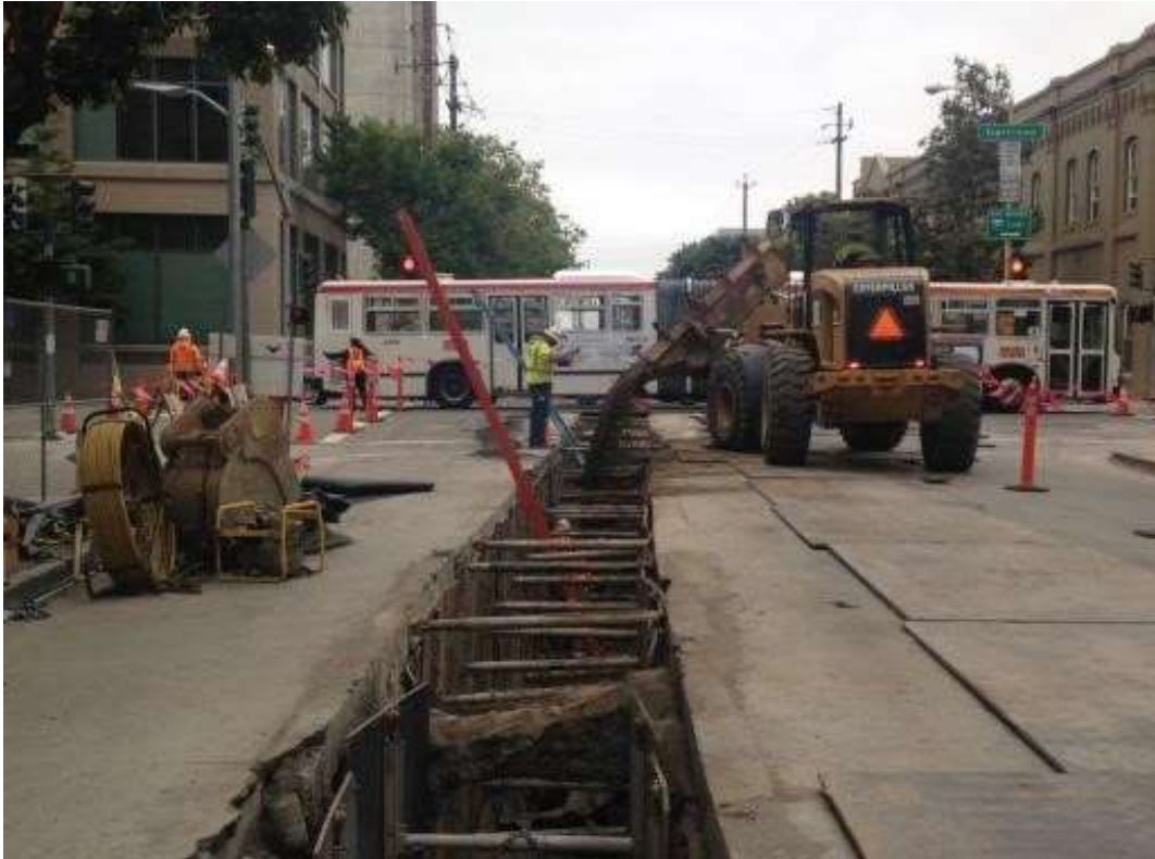
Figure 1 – Backfilling of duct bank on Spear Street on west side of Harrison Street. View east, May 18, 2015. Photo courtesy of PG&E.
