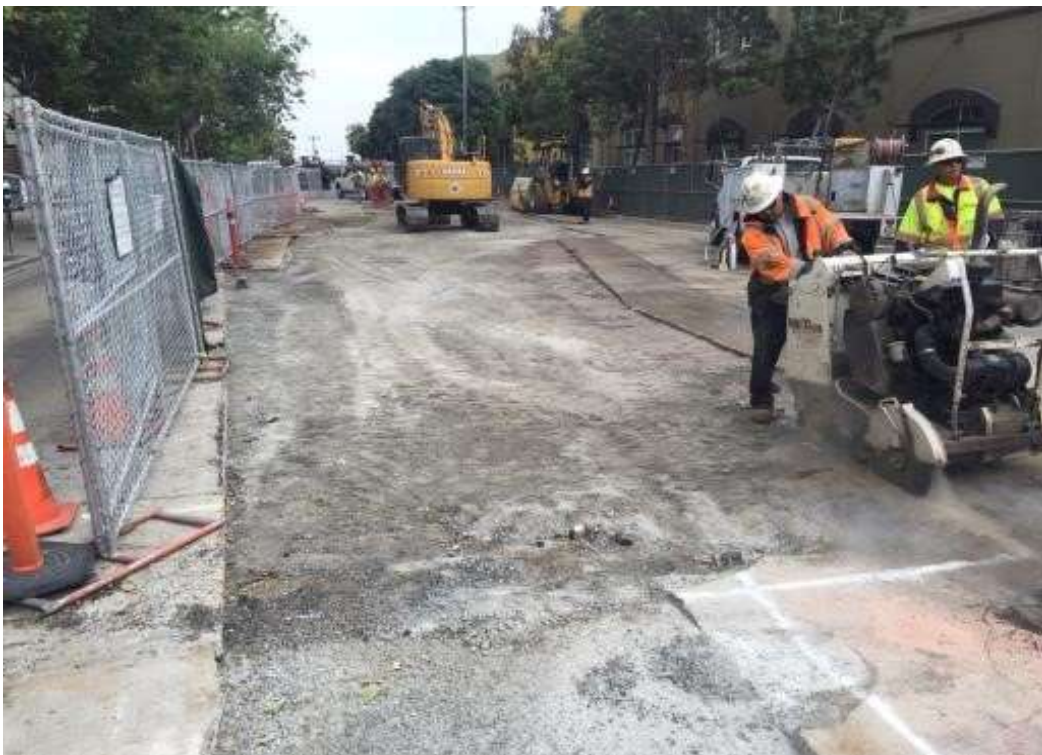
Figure 2 – Saw cutting pavement on Spear Street in cul-de-sac. View east, May 19, 2015. Photo courtesy of PG&E.
