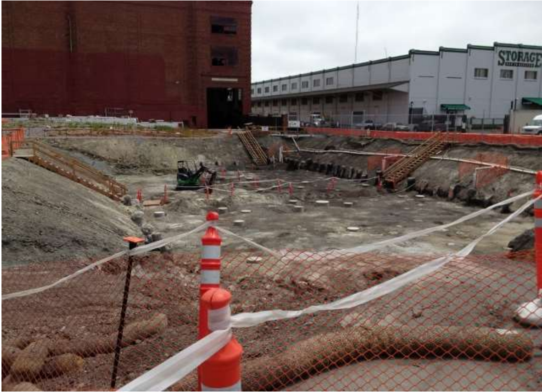
Figure 1 – Potrero Switchyard. View southeast, May 28, 2015.
