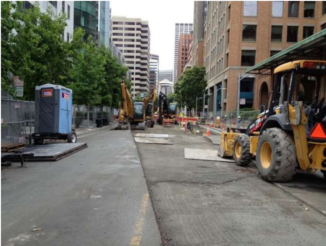
Figure 2 – Duct Bank North on Spear Street between Harrison Street and Folsom Street. View west, June 10, 2015.
