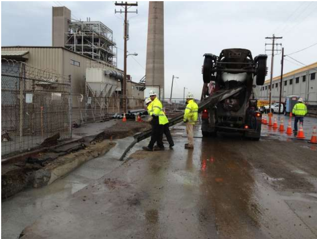
Figure 3 – Backfilling Duct Bank South with concrete on 23 rd Street. View east, June 10, 2015.
