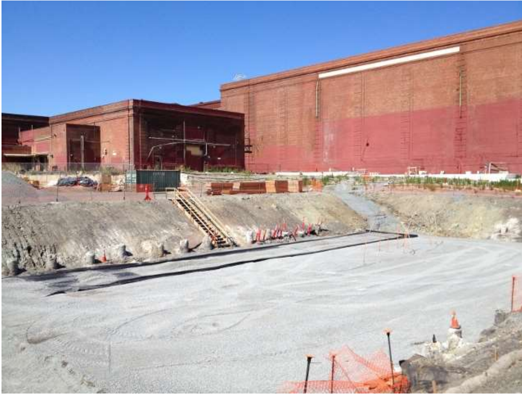
Figure 1 – Potrero Switchyard. View northeast, June 16, 2015.
