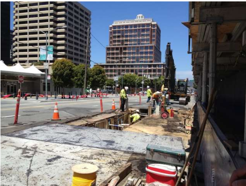
Figure 2 – Duct Bank North shoring on Folsom Street between Beale Street and Main Street. View northwest, June 16, 2015.
