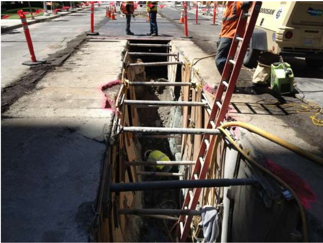
Figure 3 – Chipping away at serpentine rock in trench on Spear Street. View west, June 16, 2015.
