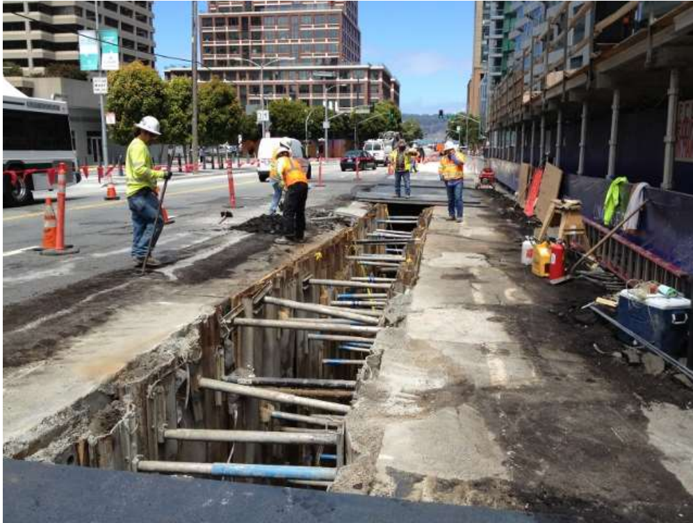
Figure 1 – Duct Bank North work on Folsom Street between Beale Street and Main Street. View north, June 22, 2015.
