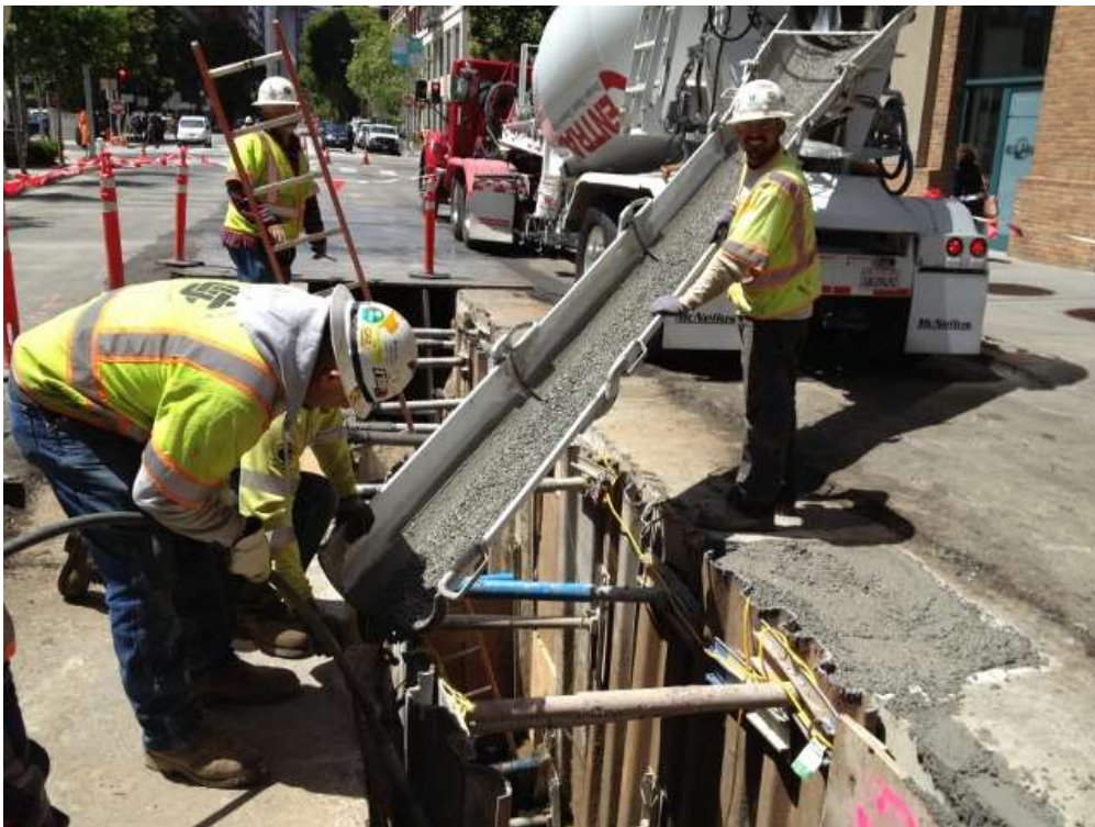
Figure 2 – Pouring cement slurry behind shoring in trench on Spear Street. View west, June 22, 2015.
