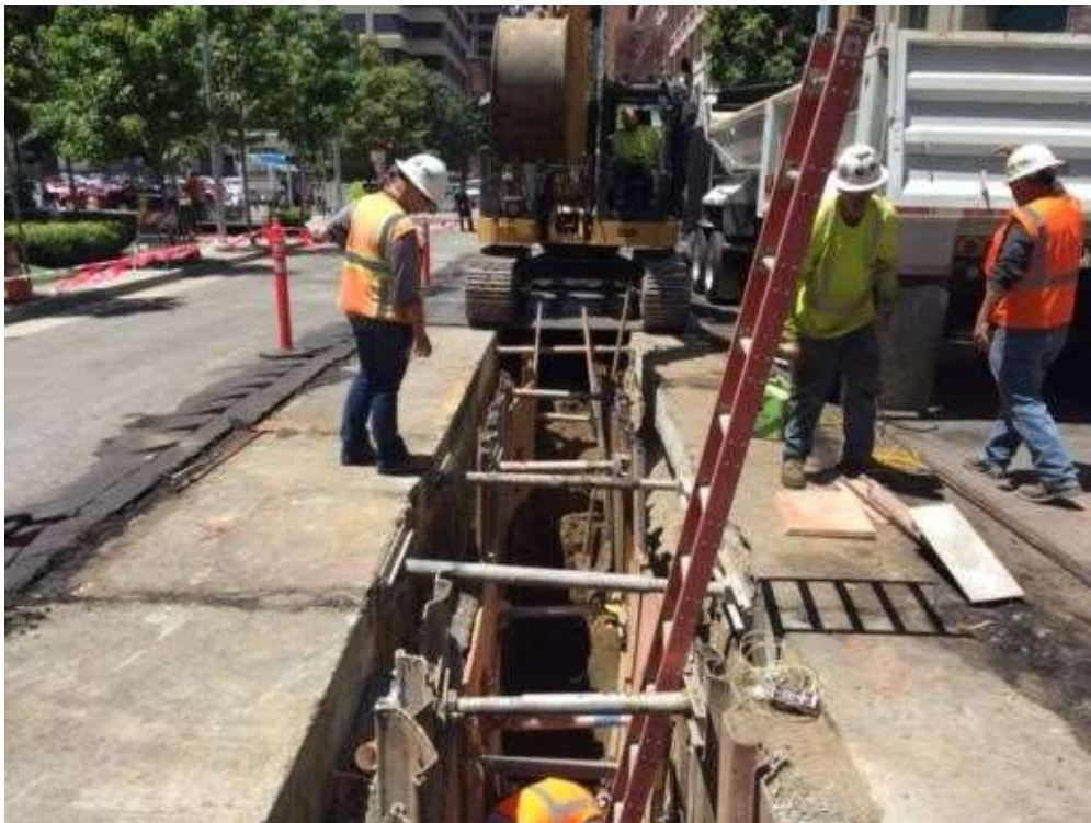
Figure 2 – Excavating duct bank trench on Spear Street. View west, June 30, 2015. Photo courtesy of PG&E.
