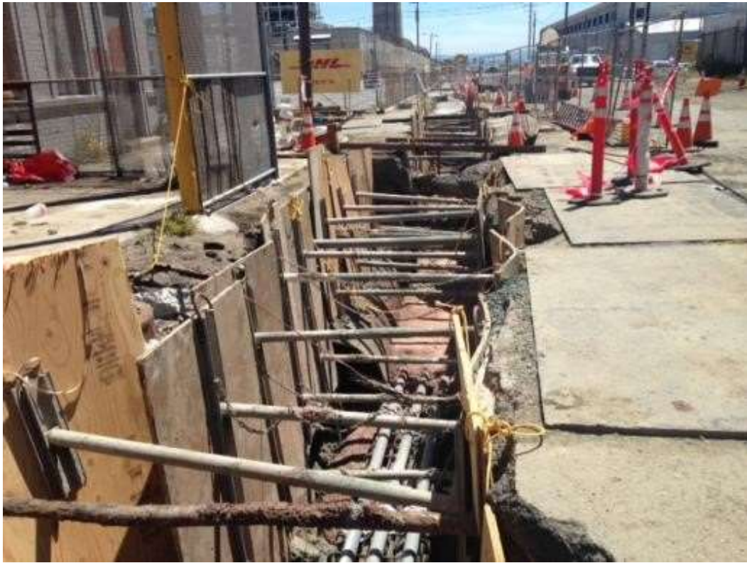
Figure 3 – Concrete slurry poured in duct bank trench on 23 rd Street. View east, June 29, 2015. Photo courtesy of PG&E.
