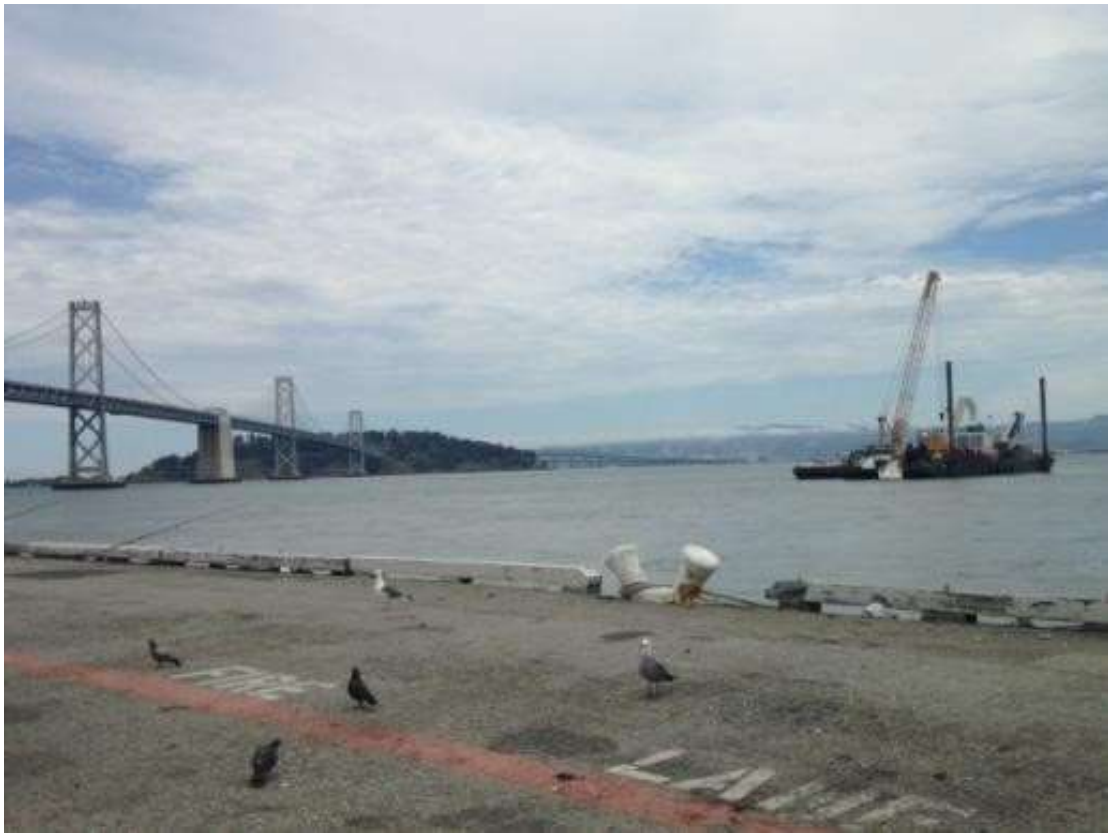
Figure 5 – Durocher positioning vessel off Pier 30/32 for submarine cable installation. View northeast, July 2, 2015. Photo courtesy of PG&E.
