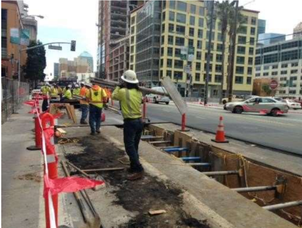
Figure 1 – Removing shoring from trench on Folsom Street. View south, July 2, 2015. Photo courtesy of PG&E.
