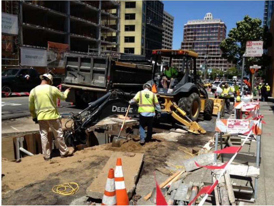
Figure 1 – Duct Bank North work on Folsom Street between Fremont Street and Zeno Place. View northwest, July 16, 2015.
