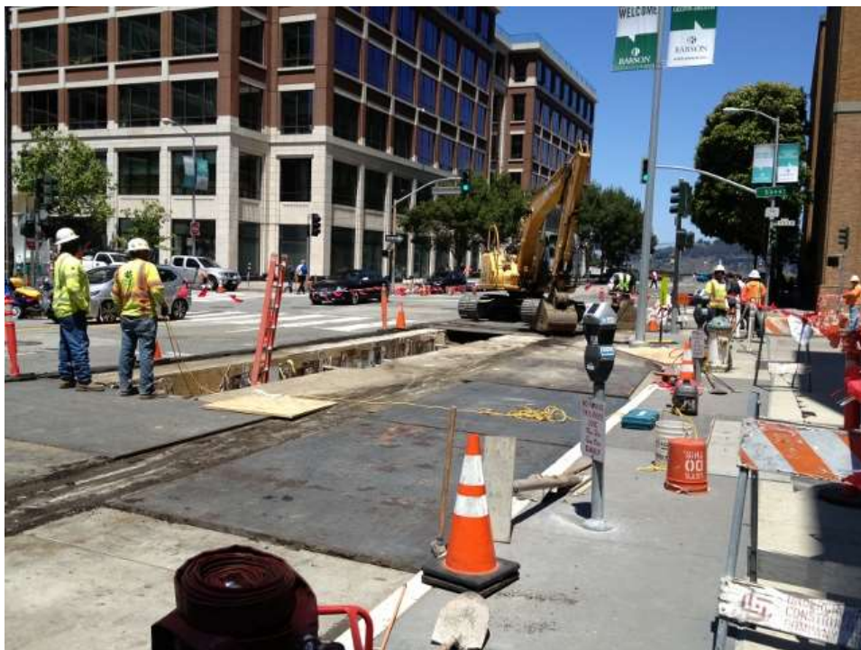
Figure 2 – Duct bank work on Folsom Street near Spear Street. View north, July 16, 2015.
