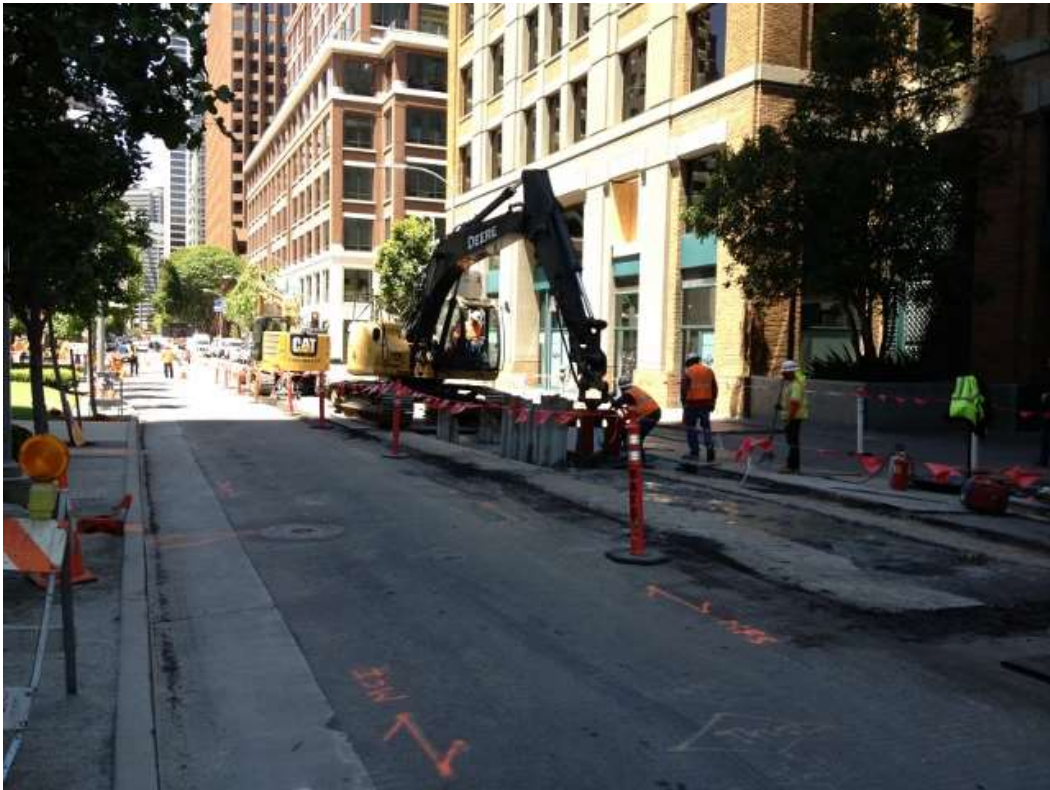
Figure 3 – Crews pouring slurry and removing shoring on Spear Street on west side of vault. View northwest, July 16, 2015.
