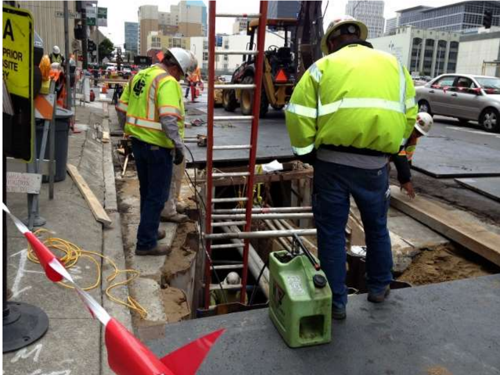
Figure 1 – Duct Bank North work on Folsom Street between Fremont Street and Zeno Place. View southwest, July 21, 2015.
