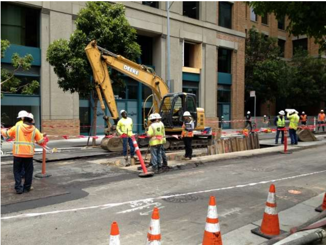
Figure 3 – Excavating duct bank trench on Spear Street on west. View north, July 21, 2015.
