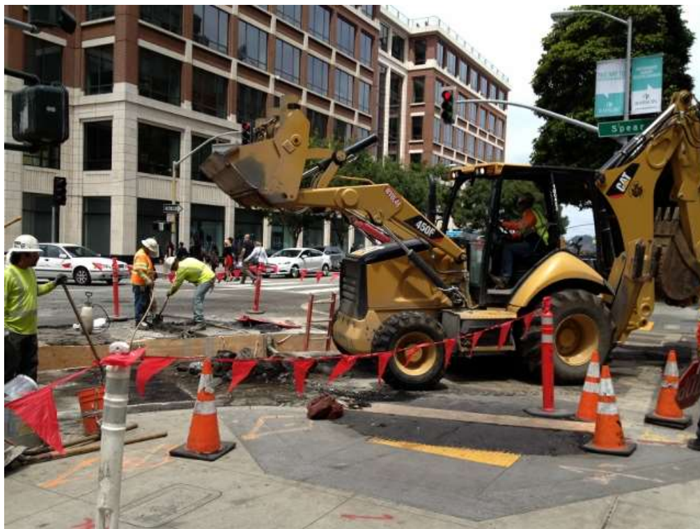
Figure 2 – Duct bank work on Folsom Street near Spear Street. View northwest, July 21, 2015.
