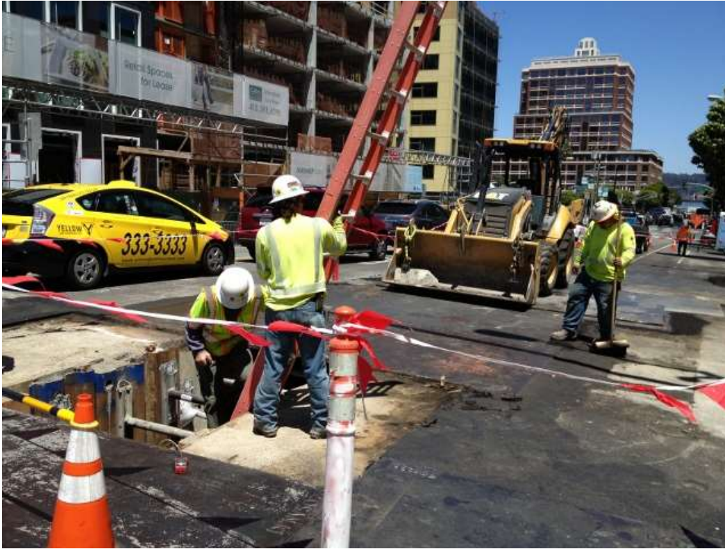
Figure 1 – Duct Bank North work on Folsom Street between Fremont Street and Zeno Place. View northwest, July 29, 2015.
