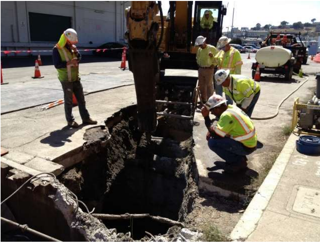
Figure 3 – Excavating duct bank trench around the Station A feature on 23 rd Street. View west, July 29, 2015.
