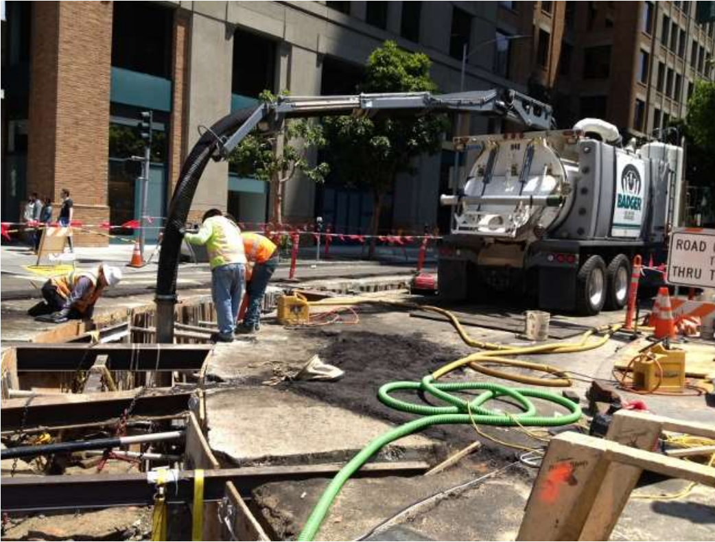
Figure 1 – Duct Bank North work on Spear Street removing saturated sandy soil from the trench with a vac-truck. View northeast, August 7, 2015.
