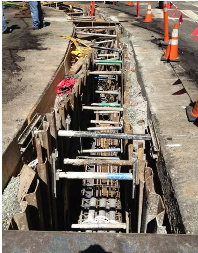
Figure 3 – Installing rebar and conduit in trench on Spear Street near Folsom Street. View west, August 14, 2015.
