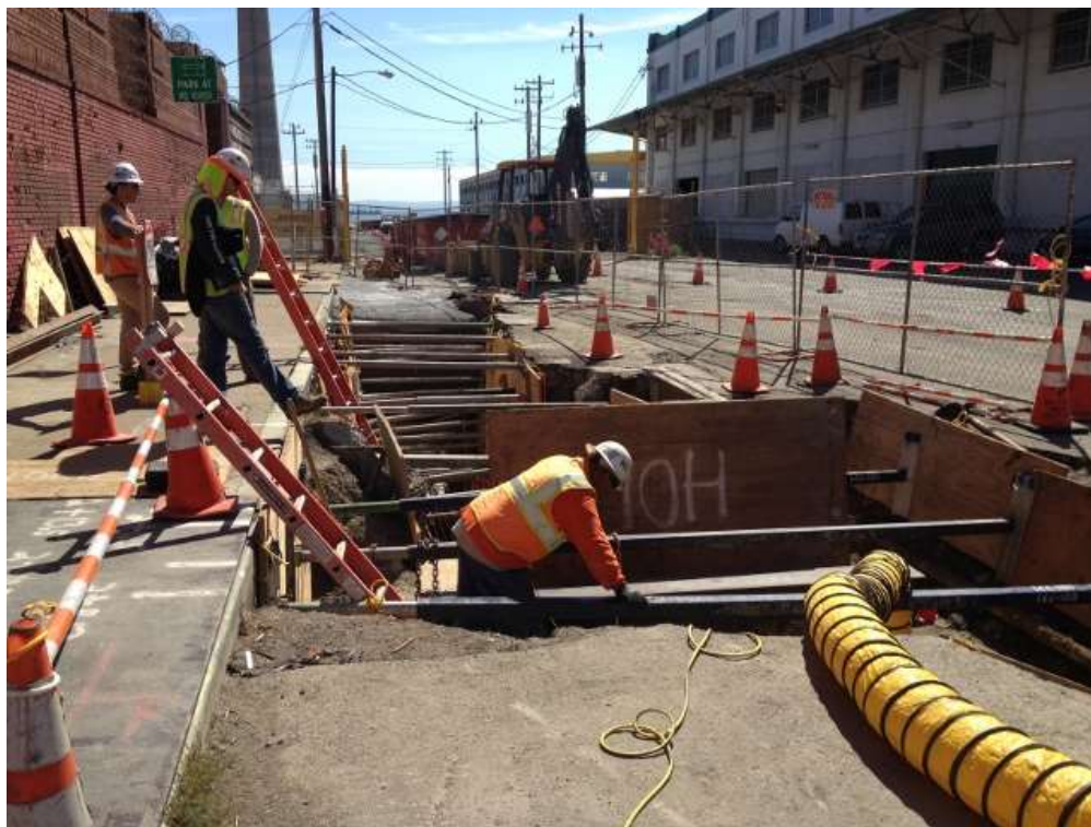
Figure 4 – Excavating the duct bank trench on 23 rd Street and working around the Station A feature. View east, August 14, 2015.
