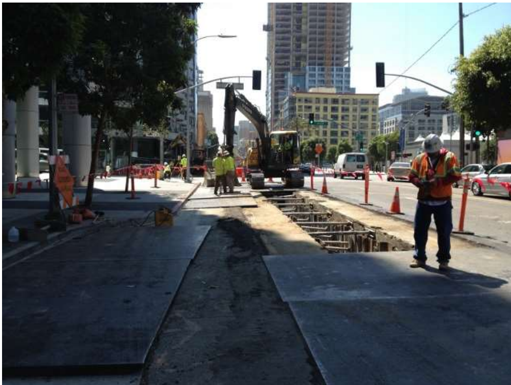
Figure 2 – Excavating duct bank trench on Folsom Street between Main and Spear Streets. View south, August 25, 2015.
