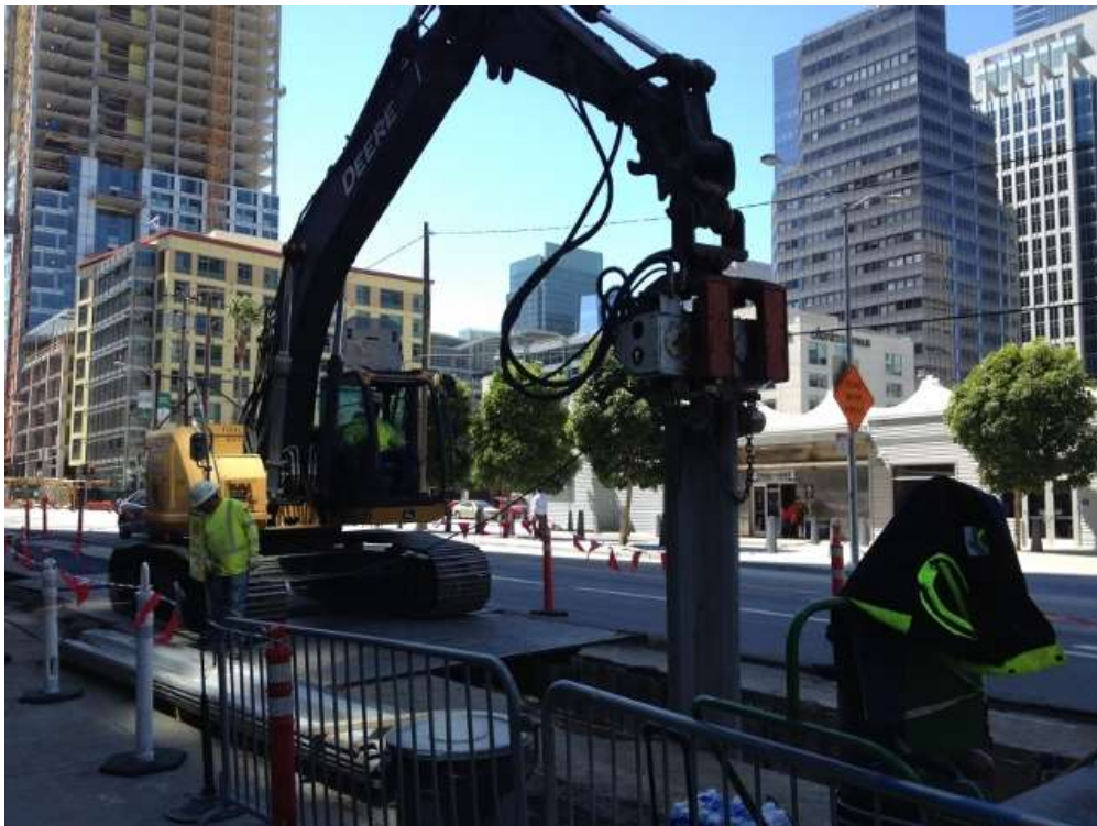
Figure 2 – Installing shoring in duct bank trench on Folsom Street between Beale and Main Streets. View southwest, September 1, 2015.
