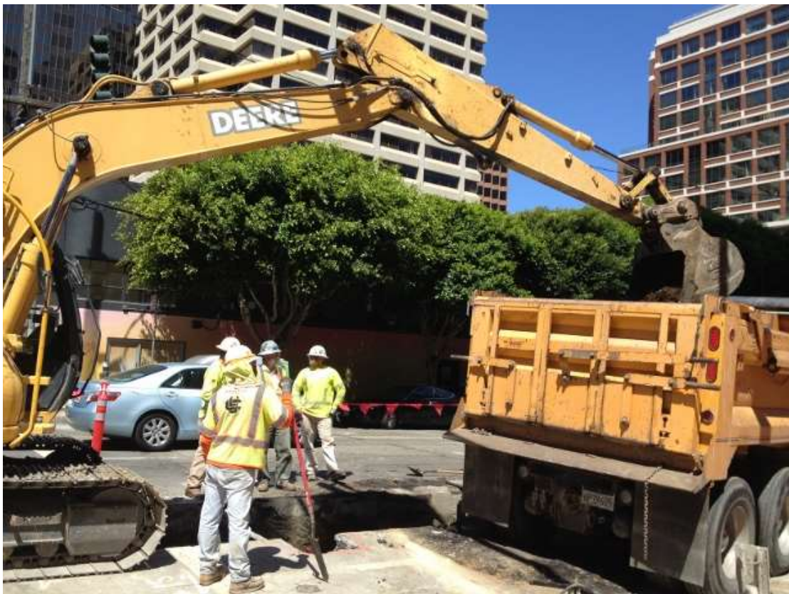
Figure 3 – Excavating duct bank trench on Folsom Street between Main and Spear Streets. View west, September 1, 2015.
