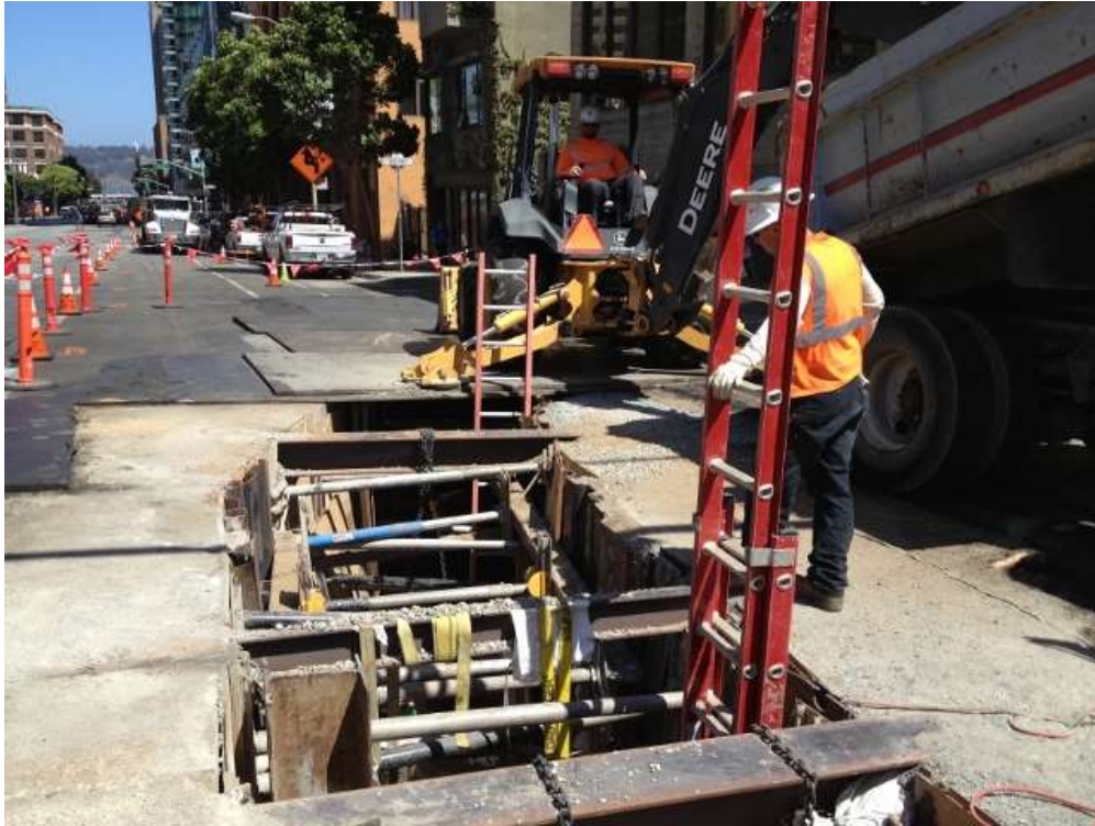
Figure 1 – Excavating duct bank trench on Folsom Street between Fremont and Beale Streets. View north, September 1, 2015.
