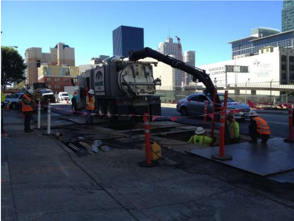
Figure 1 – Excavating the duct bank trench with a Vac-truck on Folsom Street between 1 st Street and Fremont Street. View southwest, October 1, 2015.
