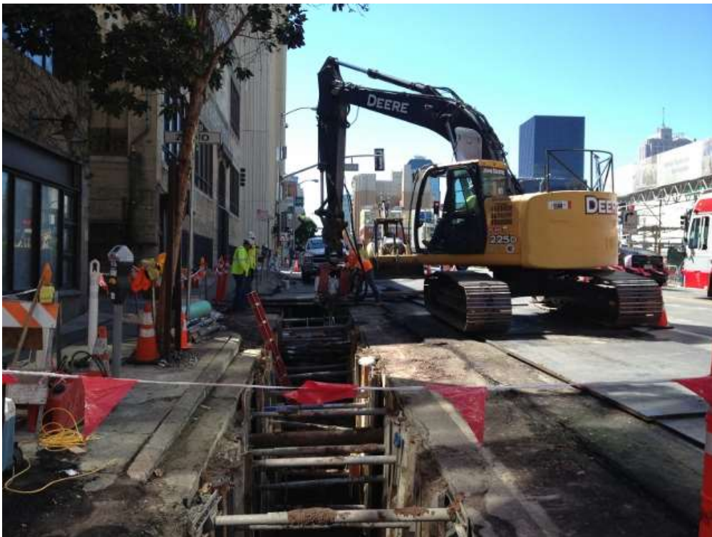
Figure 2 – Removing shoring from trench on Folsom Street between Fremont and Beale Streets. View south, October 1, 2015.
