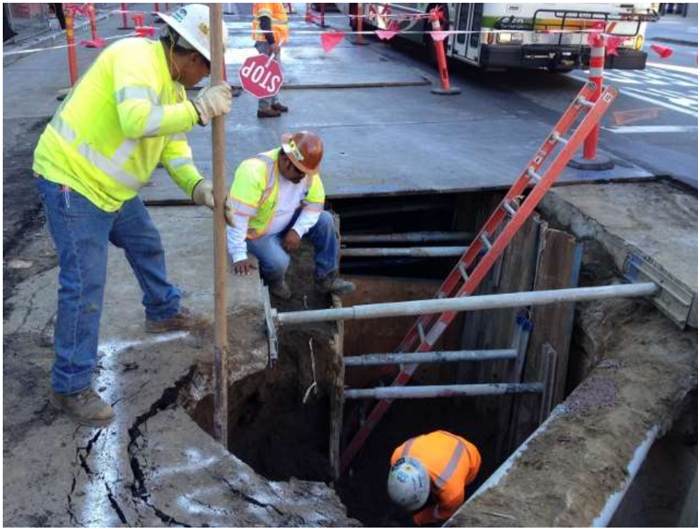
Figure 3 – Potholing for utilities on Folsom Street at Main Streets View southwest, October 1, 2015.
