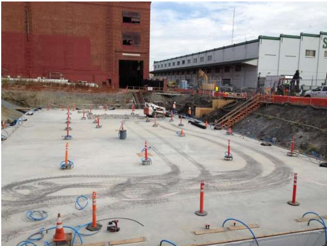
Figure 4 – Crews installing drains around the GIS building foundation at the Potrero Switchyard. View southeast, October 15, 2015.
