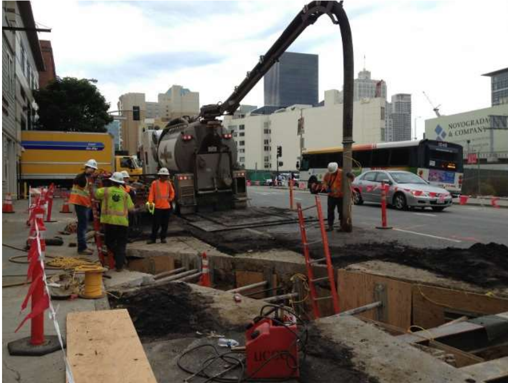
Figure 1 – Excavating the duct bank trench with a Vac-truck on Folsom Street just outside the new Embarcadero Substation addition. View southwest, October 15, 2015.
