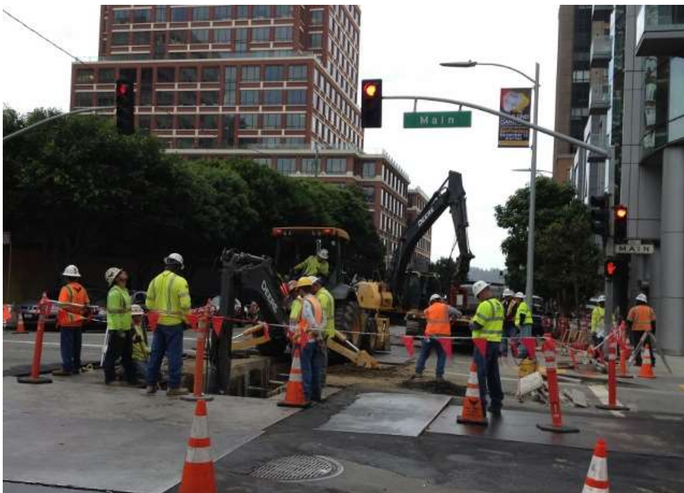
Figure 2 – Excavating trench and installing shoring on Folsom Street at Main Street. View north, October 15, 2015.
