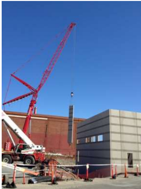
Figure 4 – Crane setting GIS building wall panels at Potrero Switchyard. View east, October 29, 2015.
