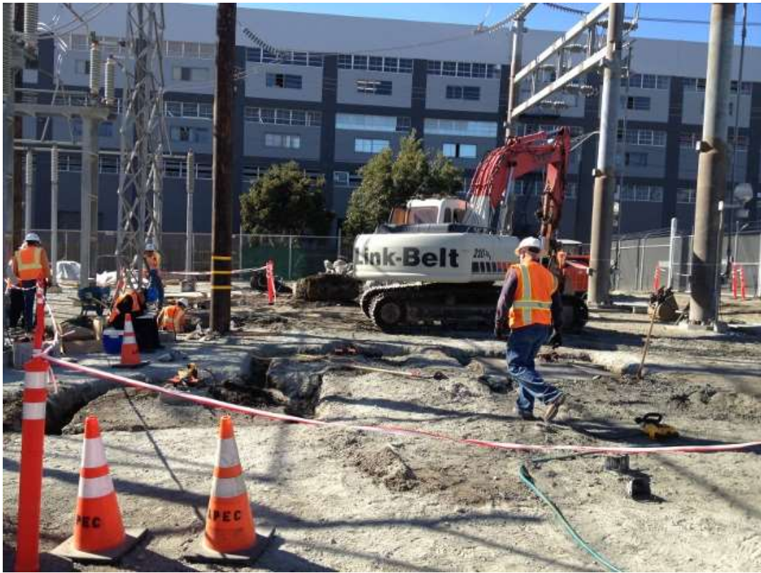
Figure 5 – Crews excavating foundations in substation adjacent to Potrero Switchyard. View west, October 29, 2015.
