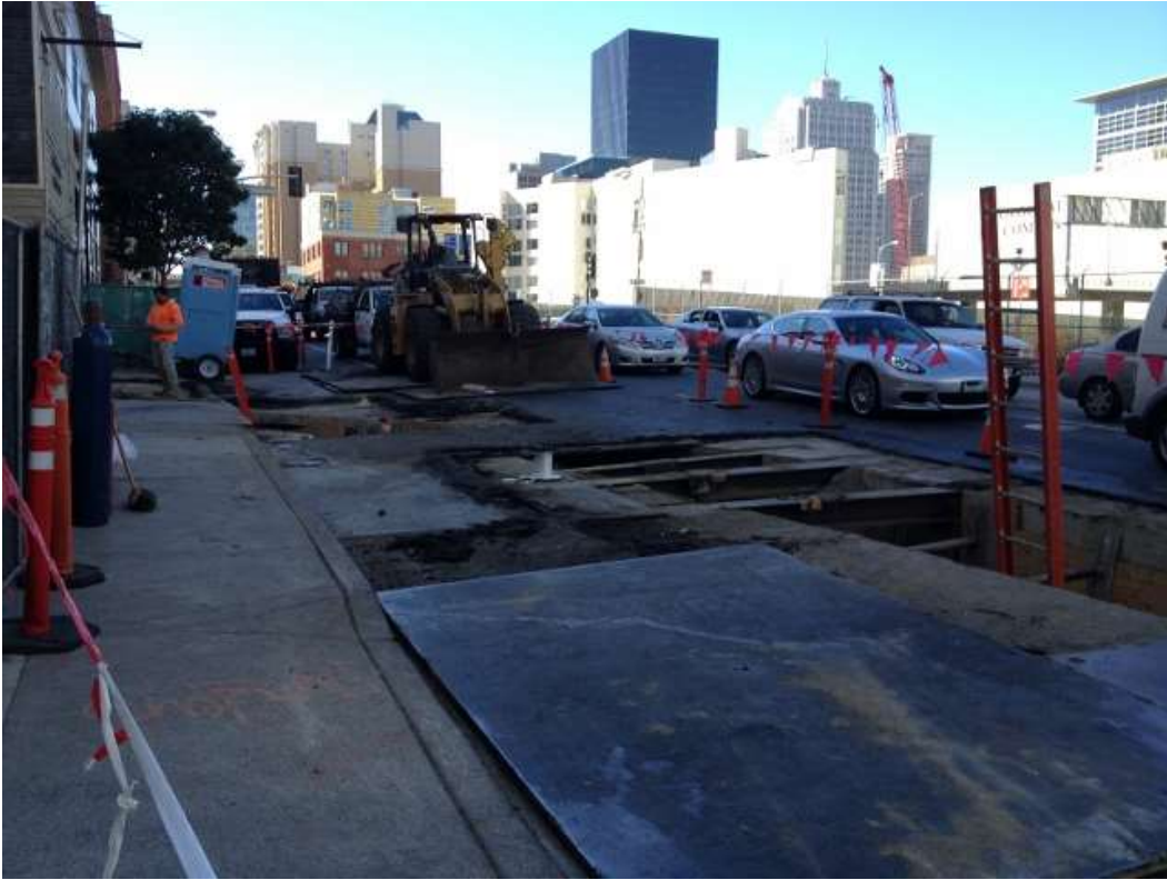
Figure 1 –Removing shoring on Folsom in front of the Embarcadero Substation. View southwest, October 29, 2015.
