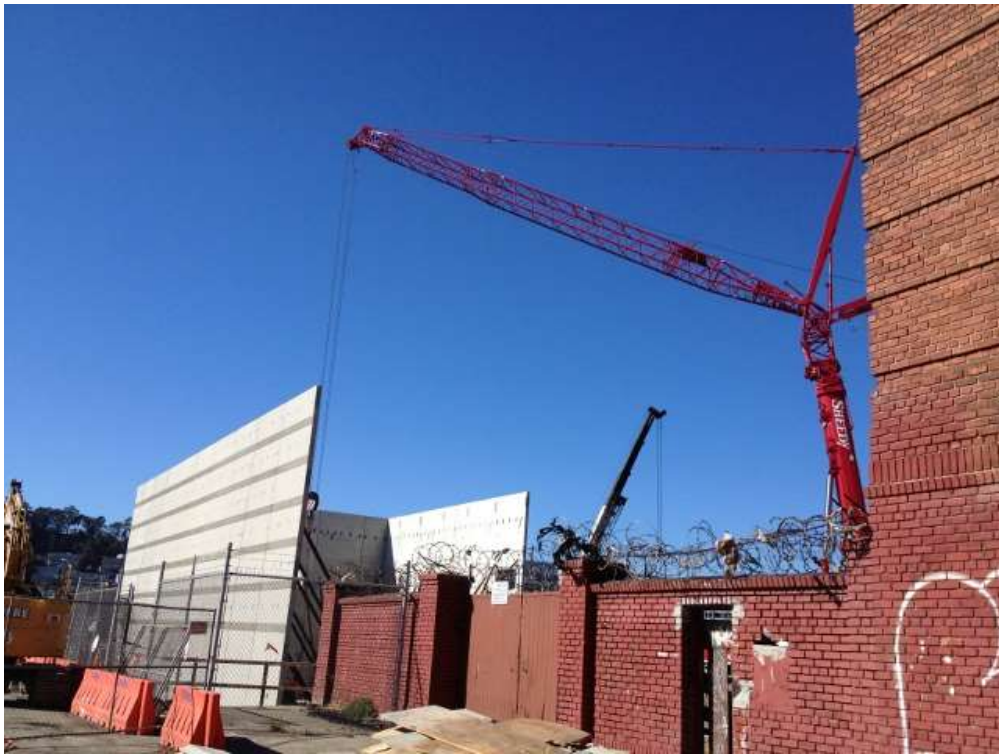
Figure 3 – GIS building wall panels being set by crane at Potrero Switchyard. View northwest, October 29, 2015.
