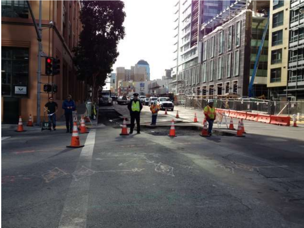
Figure 1 – Preparing to pour cement base on Folsom Street between Fremont and Beale Streets. View south, November 17, 2015.
