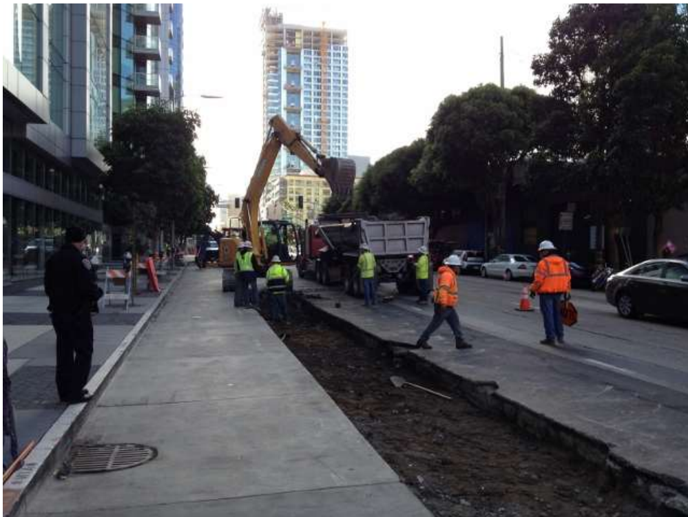
Figure 2 – Excavating pavement on Folsom Street between Main and Spear Streets. View south, November 17, 2015.
