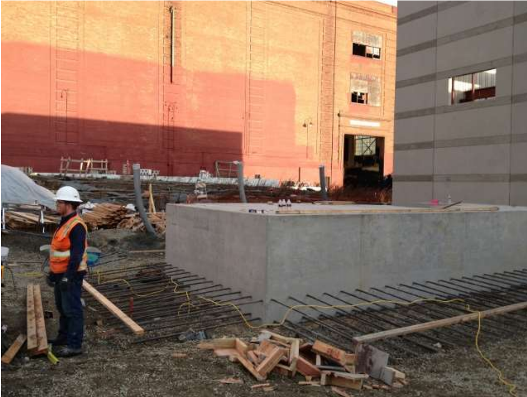
Figure 1 – Transformer pad in Potrero Switchyard. View southeast, December 11, 2015.
