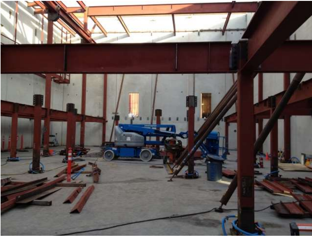
Figure 3 – GIS building at Potrero Switchyard. View east, December 11, 2015.
