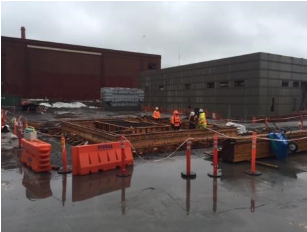
Figure 4 – Crews working on Reactor Pad in Potrero Switchyard. View southeast, December 21, 2015. Photo courtesy of PG&E.
