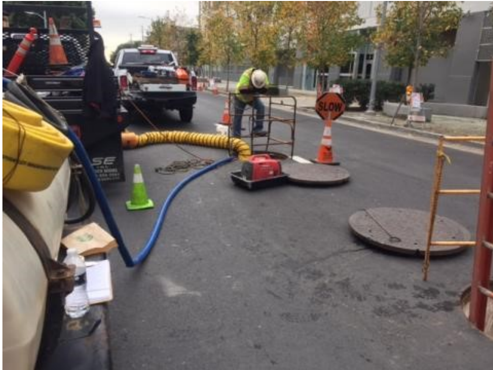
Figure 1 – Crew working in transition vault on Spear Street. View east, December 30, 2015. Photo courtesy of PG&E.
