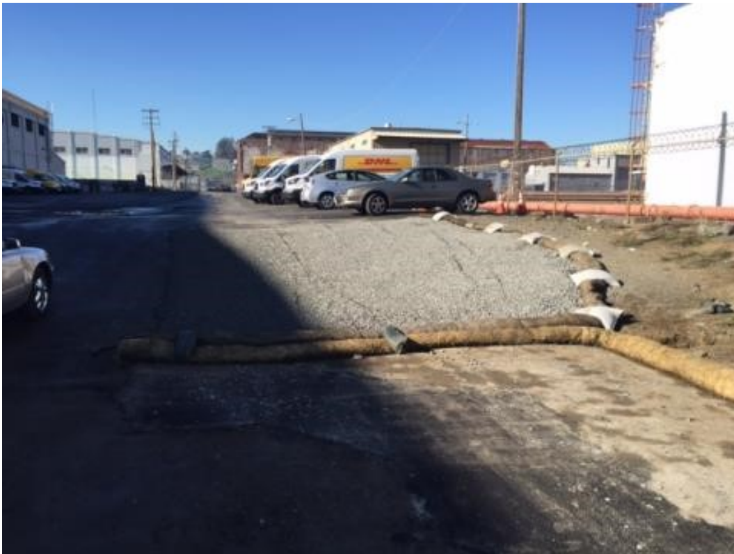
Figure 3 – Rock installed on slope at east end of 23 rd Street. View west, December 29, 2015. Photo courtesy of PG&E.
