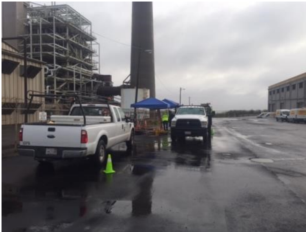
Figure 2 – Crew working in transition vault on 23 rd Street. View northeast, December 22, 2015. Photo courtesy of PG&E.
