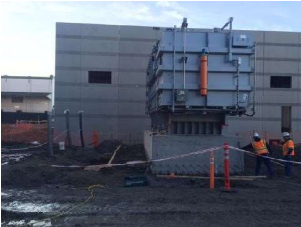
Figure 3 – APEC installing grounding cable at the transformer pad in the Switchyard. View south, January 12, 2016. Photo courtesy of PG&E.
