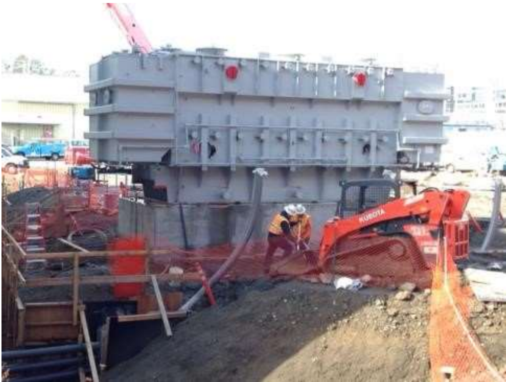
Figure 4 – APEC backfilling with base rock around the transformer pad in the Switchyard. View west, January 13, 2016. Photo courtesy of PG&E.
