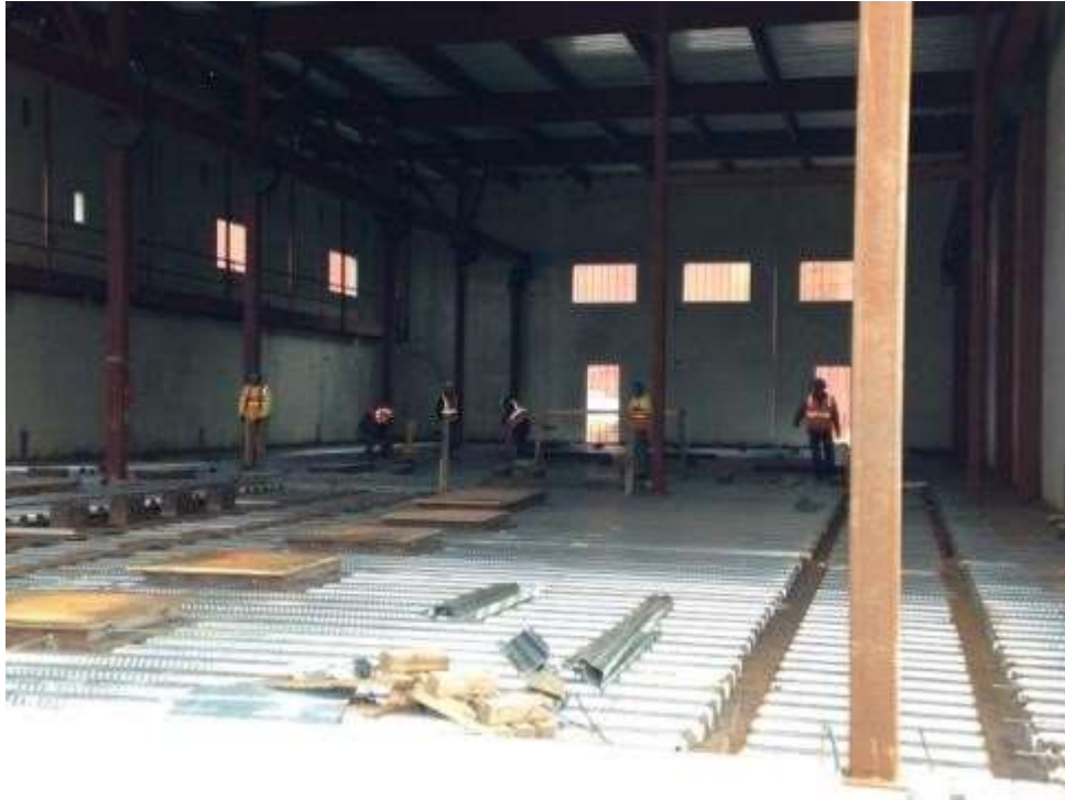
Figure 1 – B.T. Mancini installing pad decking in the GIS building in the Switchyard. View east, January 13, 2016. Photo courtesy of PG&E.
