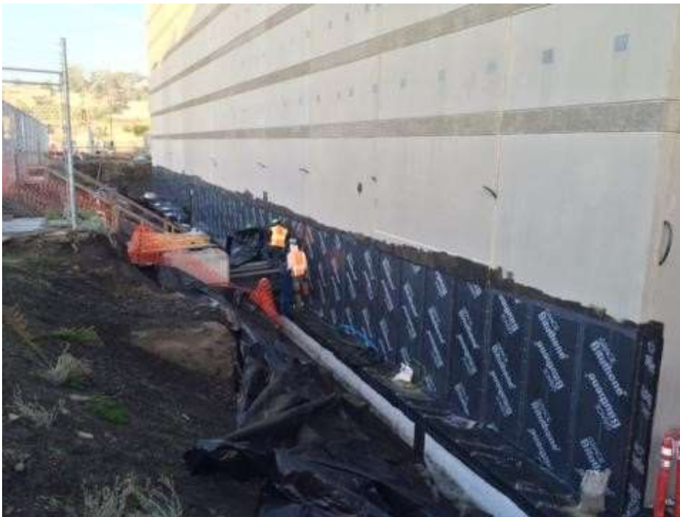
Figure 2 – ERS exposing waterproofing in preparation for re-installation on the GIS building in the Switchyard. View west, January 15, 2016. Photo courtesy of PG&E.
