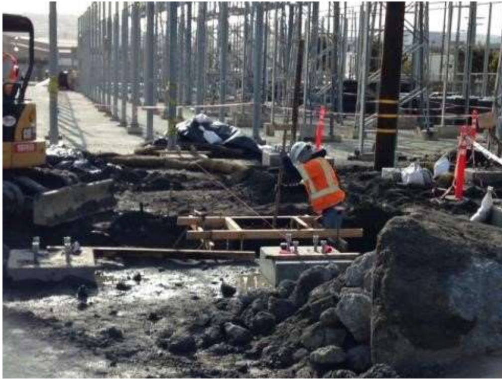
Figure 5 – APEC setting rebar cage forms in adjacent substation. View south, January 13, 2016. Photo courtesy of PG&E.
